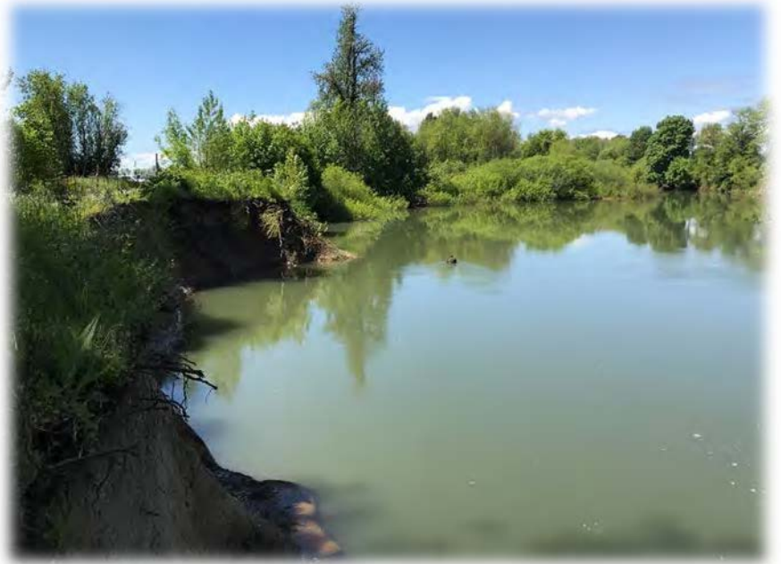
The Luckiamute River at Luckiamute State Natural Area is behaving like a natural river, migrating and meandering across the floodplain. This progression has eroded a significant portion of the bank adjacent to a road leading into the north part of the park. OPRD has determined the best course of action to address the erosion is a no action alternative, accommodating this natural river process while moving the road and parking lot out of the way. (photo by A. Berkley)
