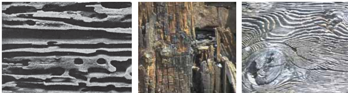
Figure 1. Wood products that are in contact with the ground or exposed to weather can be damaged by a variety of damaging insects (left), fungi (middle), and marine borers, as well as by the weather itself (right).
