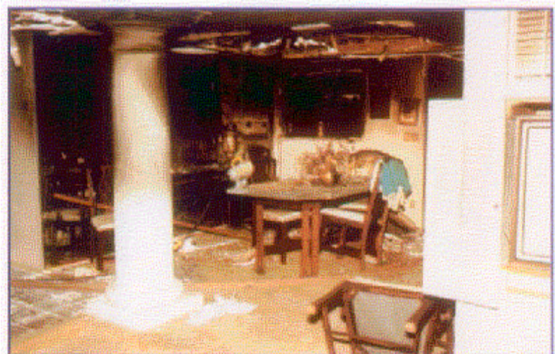
Smoke and heat damage extended throughout the living area despite the fact that the fire never extended into the area. (CS5-5)
