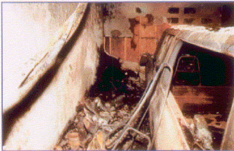
The point of origin which consisted of smoking materials in a combustible container. The interior of the garage sustained extensive damage and breached the one hour fire protection envelope. (CS5-2)
