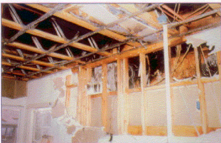
Overhead fire traveled to adjoining units through open combustible spaces. (CS3-3).
