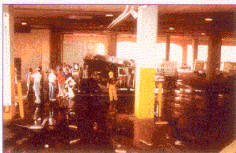
A closer view of the damage associated with the explosion. The sprinkler pipe remained intact. (CS1-6)
