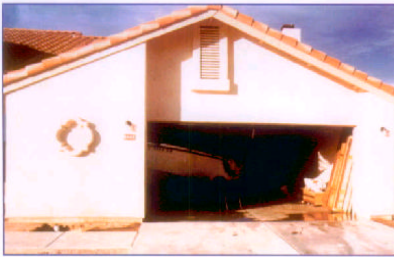
The outside view of the newly completed residence that had just experienced a garage fire. (CS4-1)
