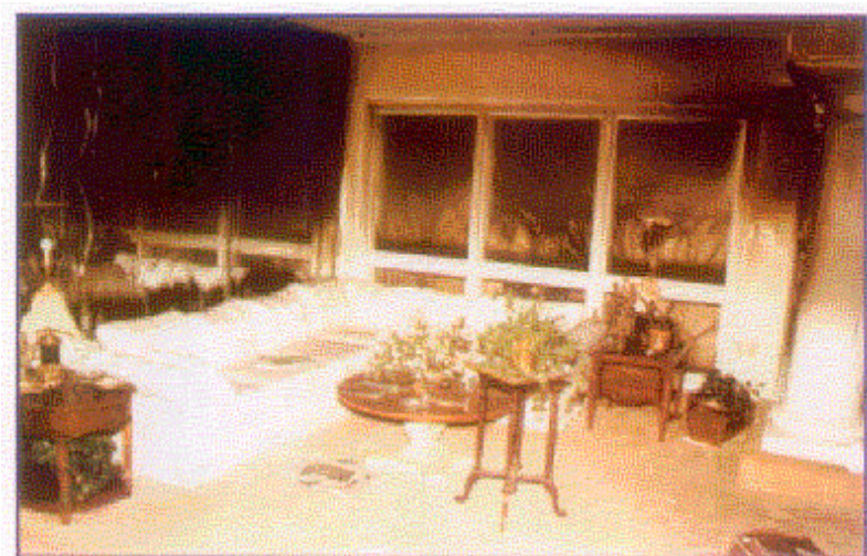
Severe smoke damage well away from the actual fire. (CS5-6)
