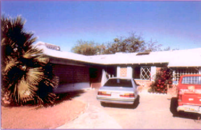
Overall view of single story, block construction, composition roof structure. Other than the ventilation hole cut by suppression crews, and burned wood at the top of the entrance, it is difficult to identify this home experienced a major interior fire. (CS9-1)
