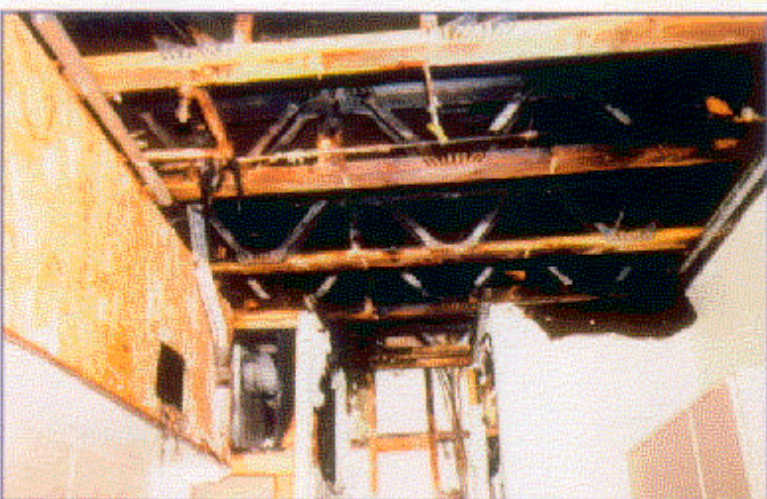
An example of rapid fire spread through an unprotected, combustible, concealed space. (CS3-6)
