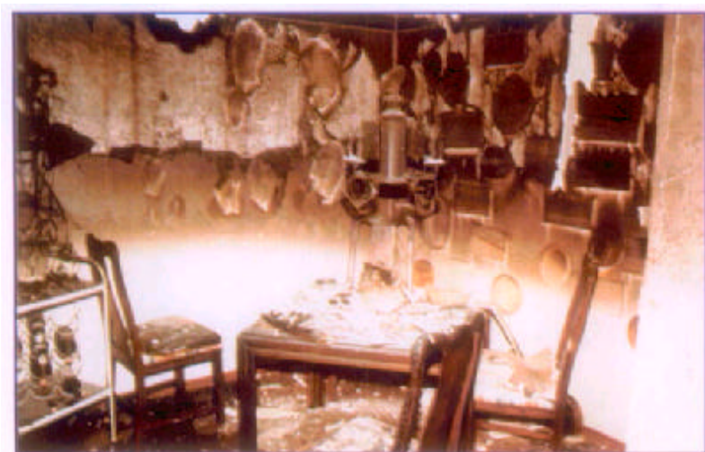
Although the fire never reached the dining area, smoke and heat damage were significant. (CS5-4)
