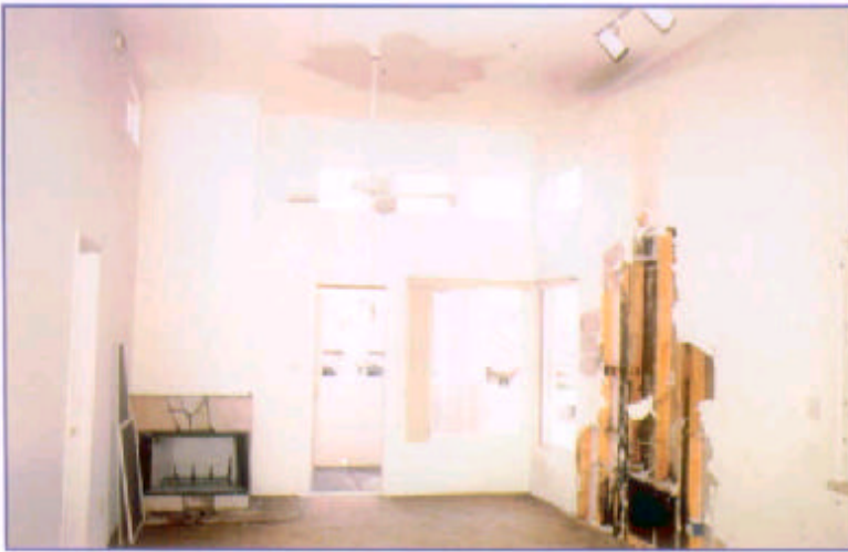
Fire extended vertically to the second floor where it activated an automatic sprinkler head. The activation helped control further spread of the fire and prevented additional structural damage. (CS3-4)
