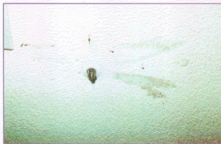
The activated sprinkler head caused only minor damage to the finish of the ceiling area. (CS6-2)
