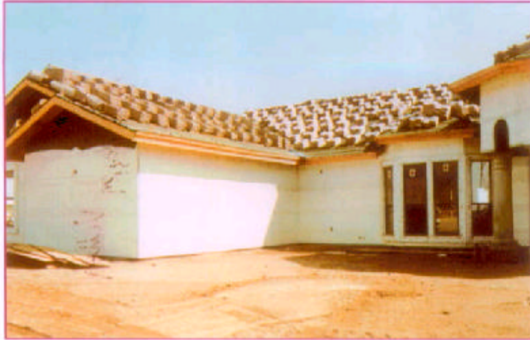
The structure in its most vulnerable state. Open framing with exposed combustible construction products throughout the
