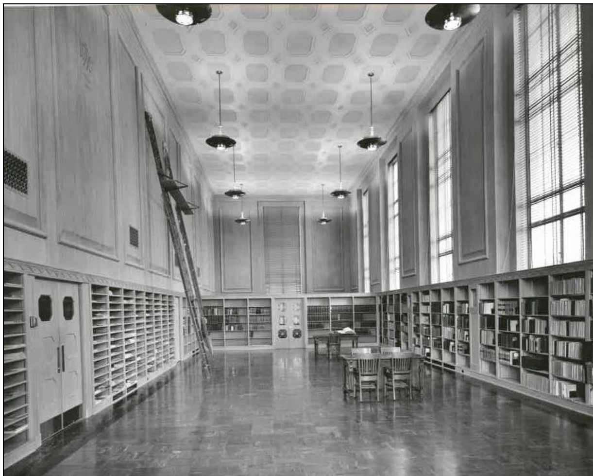
Figure 19 – Construction of State Library, reference room, February 19, 1939, shows ladder for installation of stenciled printers’ marks and cast bronze clock on panels, south side of reference room. Windows are on north side; government documents room is at west end of room behind doors with octagonal bronze grills. Three carved wood panels between shelving units on north side illustrate printing press, meadow lark, and Oregon grape.
