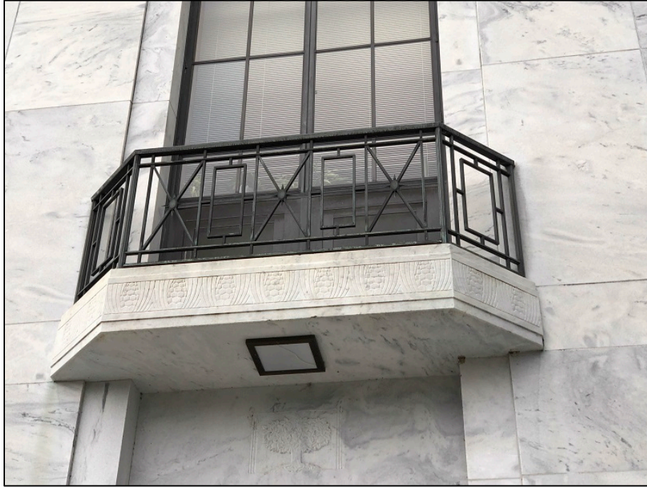
Photo 5 of 15 - OR_MarionCounty_StateLibrary_0005; balcony, pine cone and needle decoration on base of balcony, geometric rectangular and diagonal designs of balcony rail and carving of open book and tree of state library building, facing west
