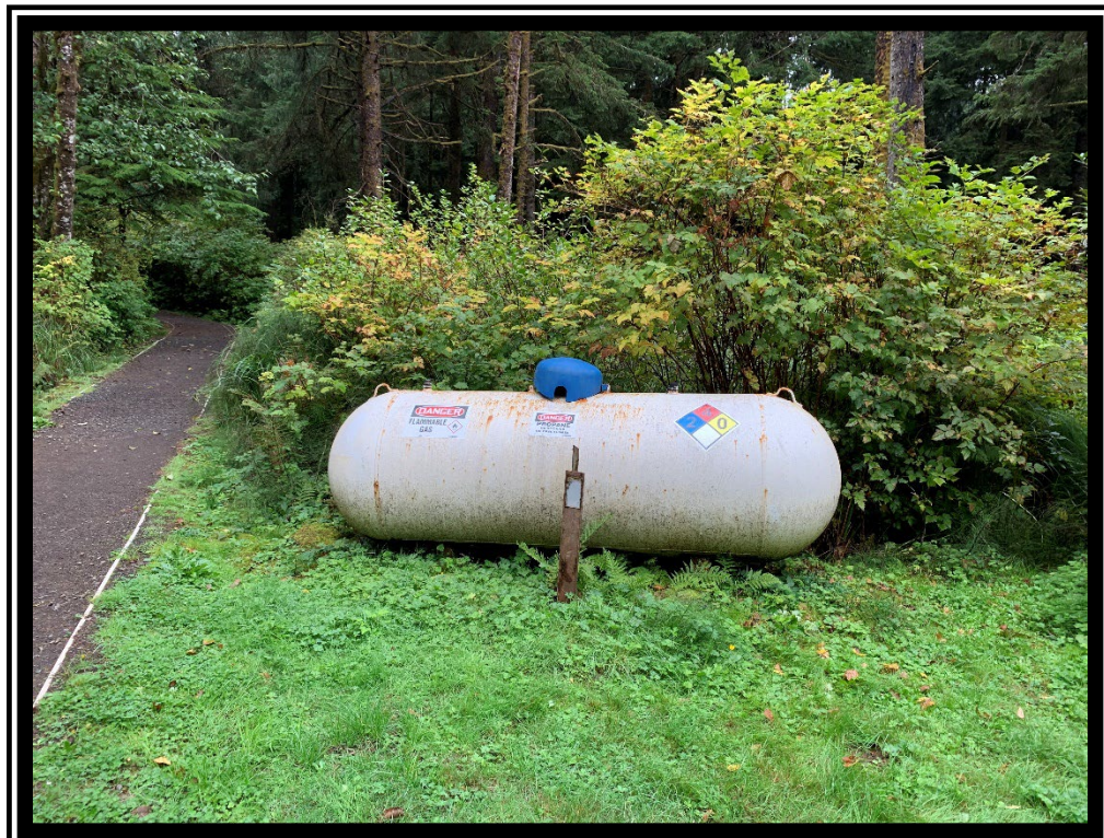
Figure 2 – Aging propane tank on instable footings.
