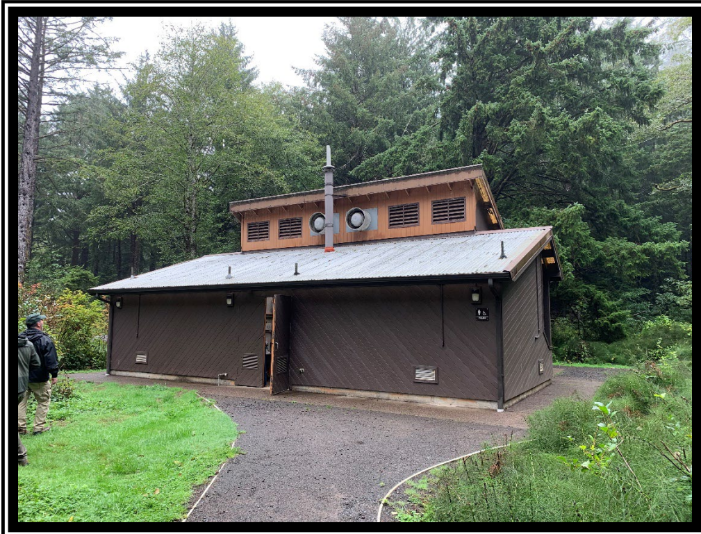
Figure 1 – Existing restroom building. Acrylic roof panels difficult/hazardous to maintain & repair
