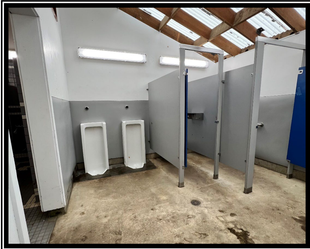
Figure 3 – End of life fixtures, difficult / hazardous to maintain.
