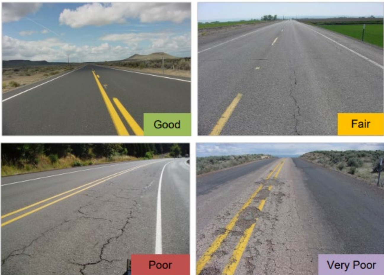
2-10 Examples of Pavement Condition Levels – Good through Very Poor
