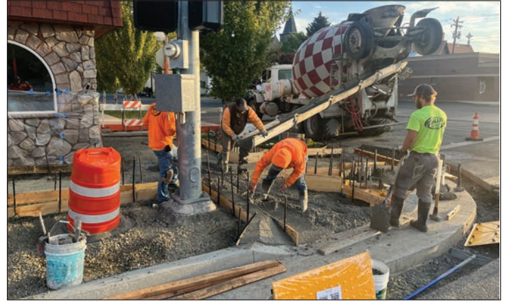
Dozens of curb ramps in Baker City and several other communities were upgraded to meet current ADA standards.
