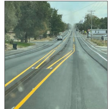
ODOT crews restriped this section of OR 207 (11th Ave.) in Hermiston to create a center turn lane.
