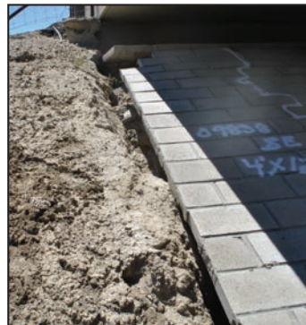
Repairs to the Benson Creek and Moores Hollow interchange bridges will be made, including fixing erosion issues like this.
