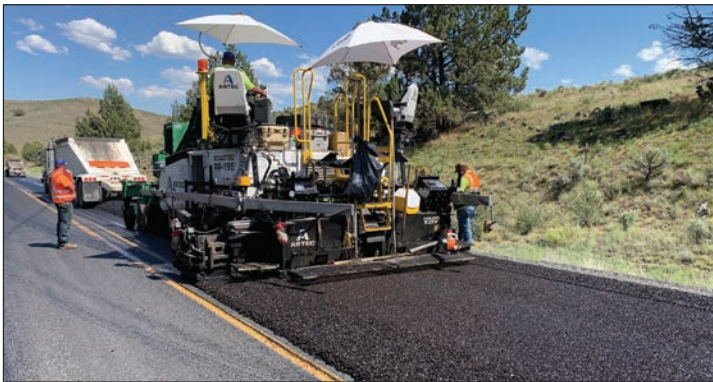
Contractors constructed a pavement overlay to sections of U.S. 20 in Malheur County.
