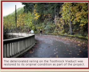
The deteriorated railing on the Toothrock Viaduct was restored to its original condition as part of the project.
