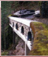
Picture right: The Eagle Creek Viaduct was damaged by a landslide and as part of the project it was repaired to its original condition.
