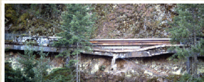
Many of the original viaducts and bridges have fallen into disrepair requiring, in some cases, major renovations and others replacement of the structure. The photograph at right is the old Eagle Creek Viaduct
