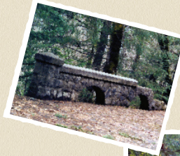
A view of the deterioration of the rubble masonry parapet walls on the Rucklee Creek Bridge.
