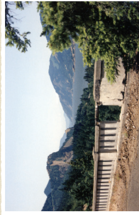
Prior to restoration, the railing in the Toothrock (above) and Ruffin Point (below) Viaducts showed marked deterioration.
