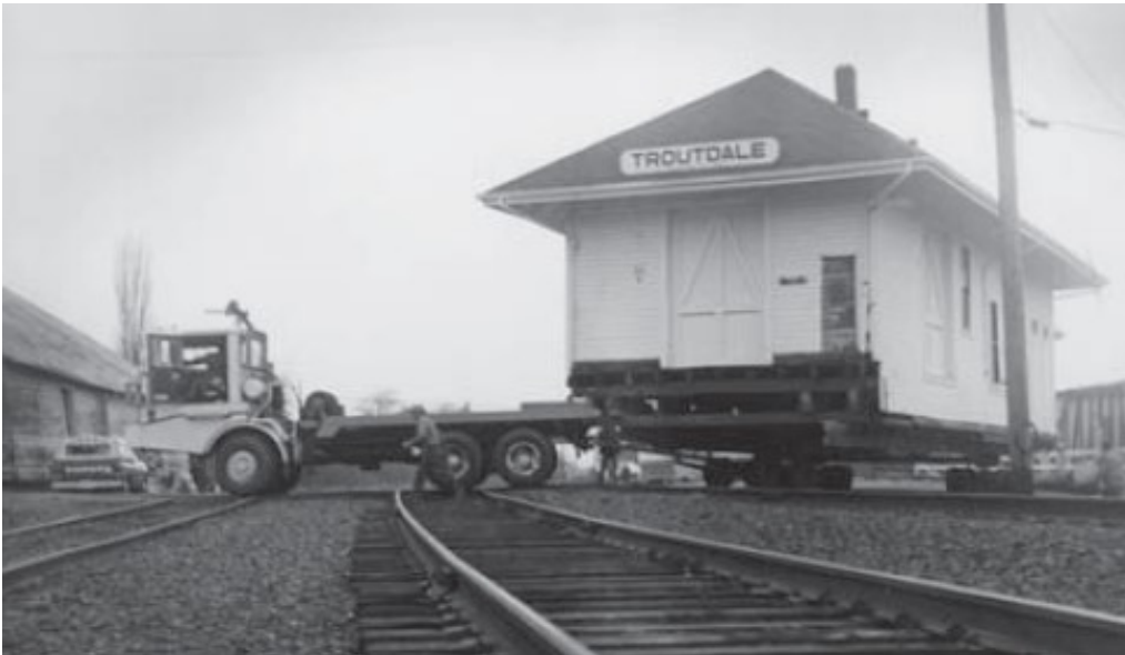
Figure 5.2 Relocation of the Troutdale depot to the north side of the right-of-way. (Troutdale Historical Society)
