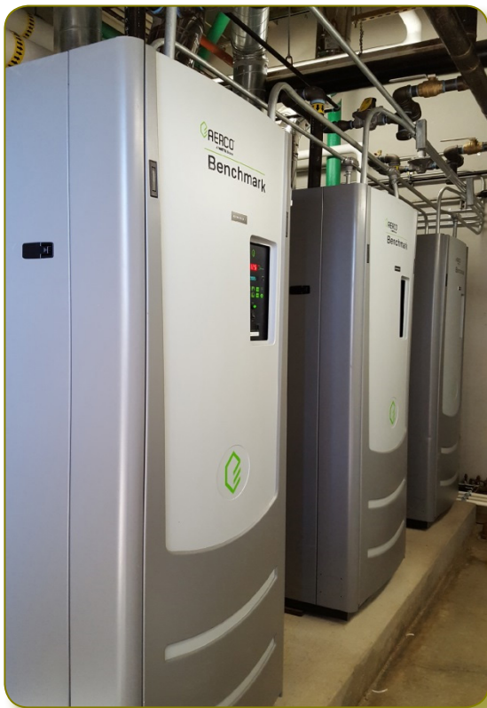
New high-efficiency condensing boilers were installed at ODOT's Materials Laboratory, in Salem.
