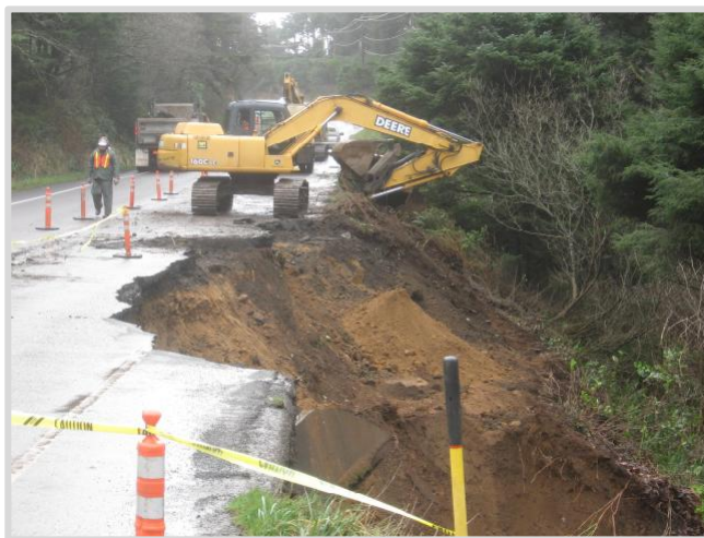
ODOT crews begin work to stabilize a slide on U.S. 101 south of Newport, January 2012.
