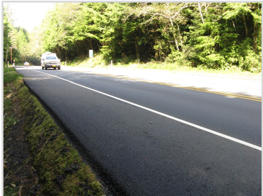
A truck travels southbound on U.S. 101 over the Falcon Cove fill slope.
