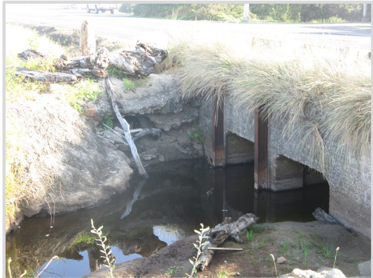
A double box culvert runs under U.S. 101 at Salt Air Creek, Rockaway Beach.
