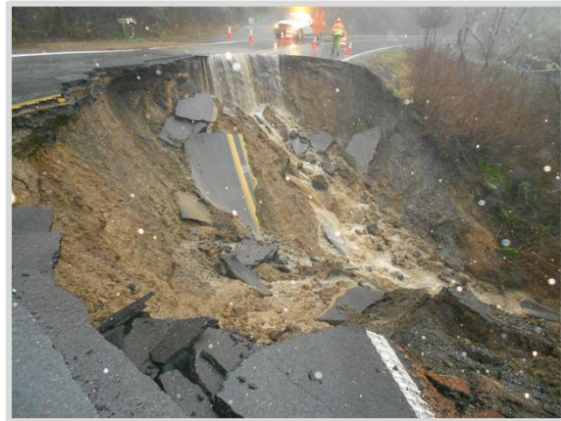
Road surface collapse on OR 255 in Curry County, January 2012.
