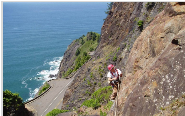
Rock fall scaling on Neahkahnie Mountain above U.S. 101 north of Manzanita.
