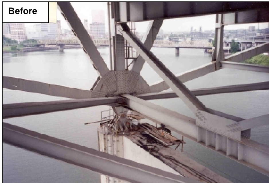
Figure 3.10A: Original Bearings on Pier #3
