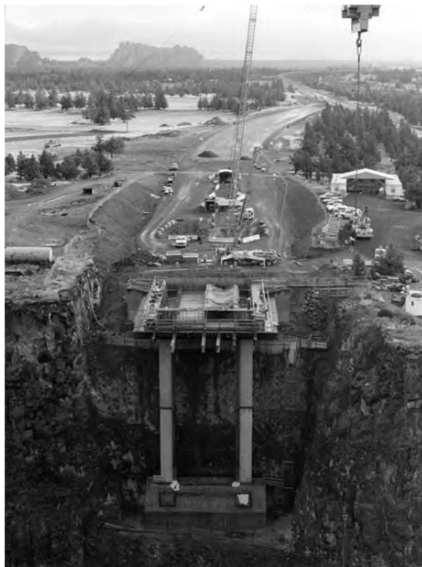
The new Crooked River Gorge Bridge will replace a bridge built in 1924 which cannot carry the increasing traffic on Highway 97.
