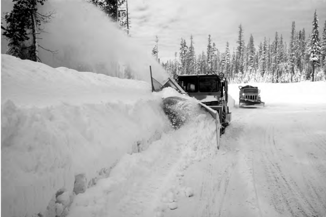
Maintenance crews respond to snow, ice, mudslides, and other weather-related conditions to keep the roads open. (Skyline Boulevard, near Mt. Bachelor)
