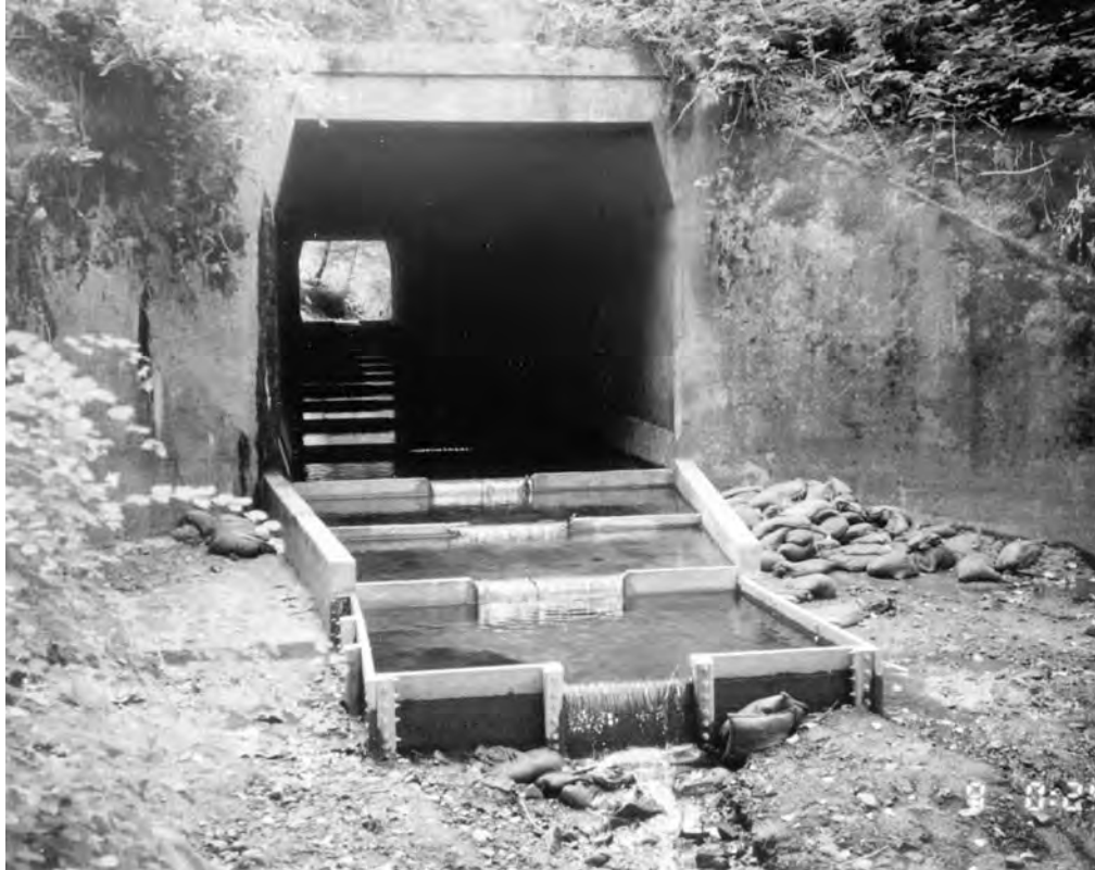
This retrofitted culvert has increased water depth, lower water velocities and a concentrated flow that will form a jump pool for endangered salmon in King Creek on the Coos Bay – Roseburg Highway (Oregon 42)
