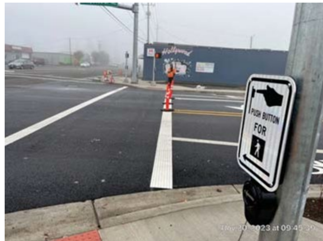
Hollywood Drive CLPA project, Marion County and City of Salem. New ADA walks, ramps, signals, left turn lane and bike lanes. -Mark Foster, Marion County
