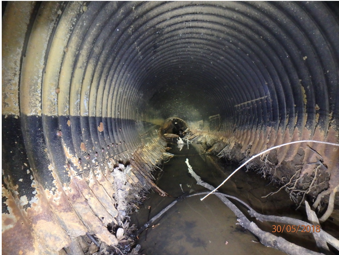
Figure 2: Photo of a critical condition corrugated metal pipe culvert with invert completely missing, rusted sides, and separated segments
