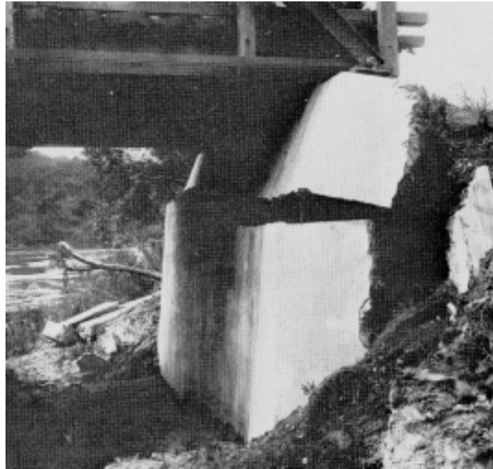
Figure 2.1: Pajaro River Bridge Damage
