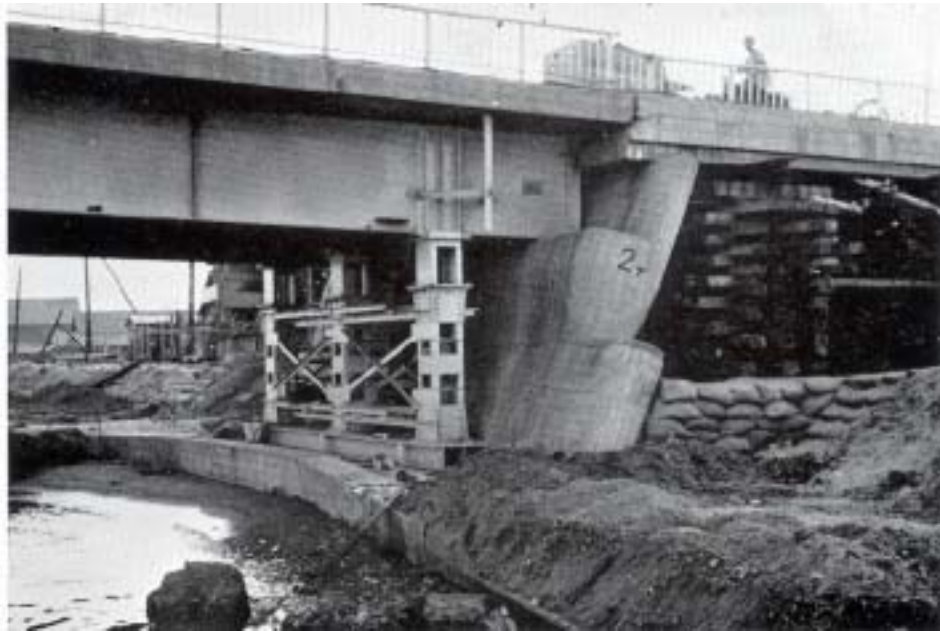
Figure 2.15: Damage to the Yachiyo Bridge
