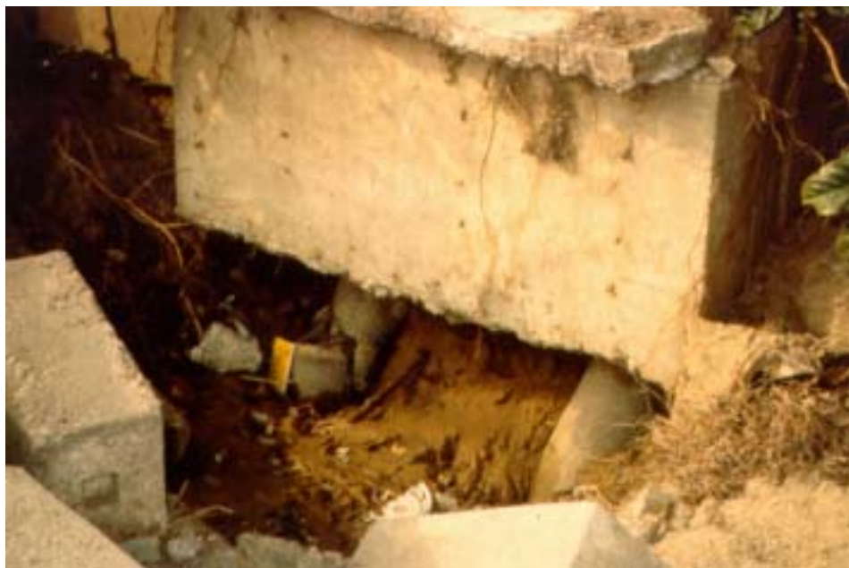
Figure 2.37: Damage to Pile Foundations near the Nadahama Ohashi Bridge
