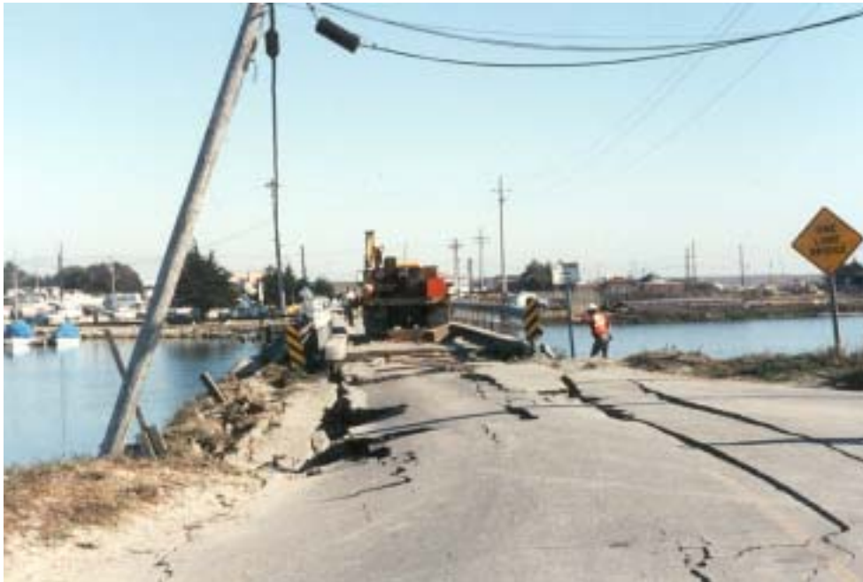
Figure 2.23: Excessive Settlement of Approach Fill
