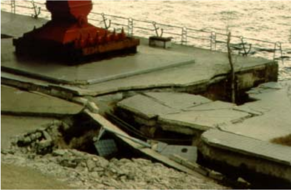
Figure 2.33: Foundation Damage at Kobe Ohashi Bridge
