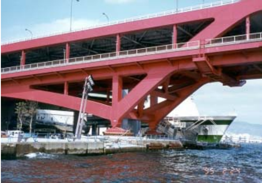
Figure 2.32: Kobe Ohashi Bridge Damage
