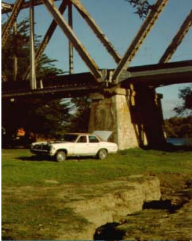
Figure 2.22: Ground Deformations Next to Railroad Bridge Pier
