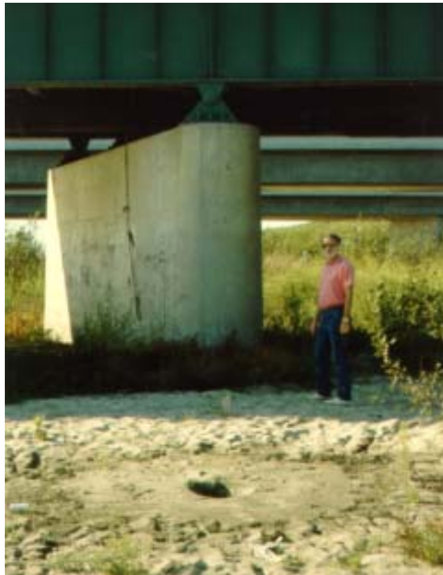
Figure 2.21: Liquefaction-induced Lateral Spreading beneath the Salinas River Highway Bridge
