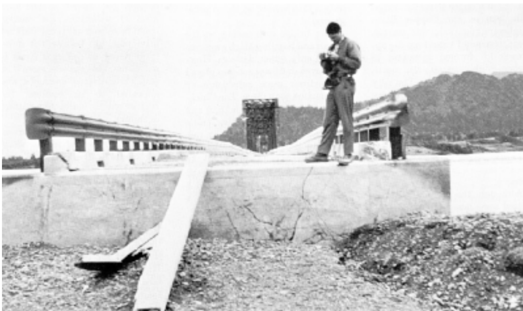
Figure 2.10(b): Post-earthquake Settlement at Copper River Bridge 334
