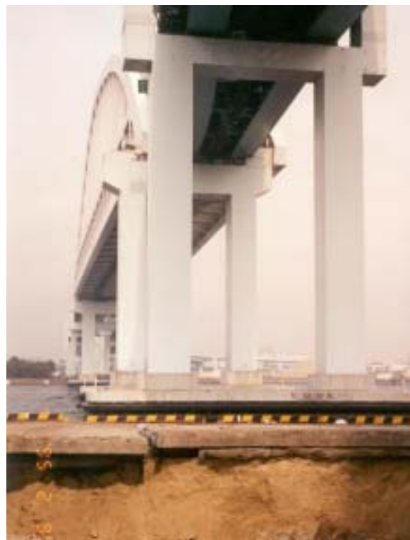
Figure 2.31: Displacements to Bridge Foundations at Rokko Ohashi Bridge
