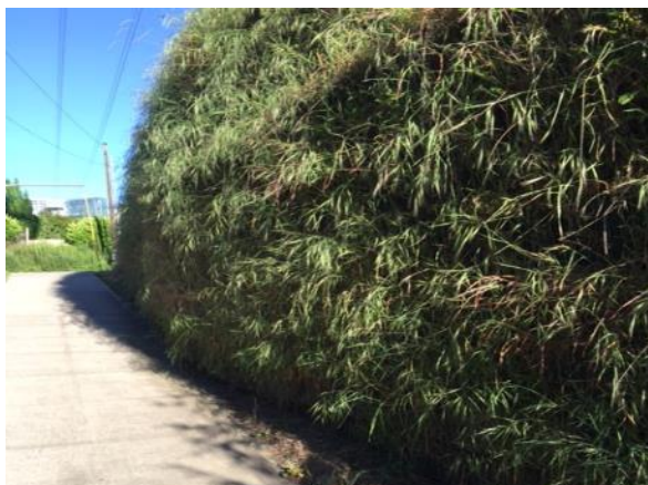
This planted gabion wall is comprised of soil enclosed in geotextile fabric
