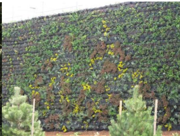
Green wall of soil filled geotextile fabric bags is tied back into the slope
