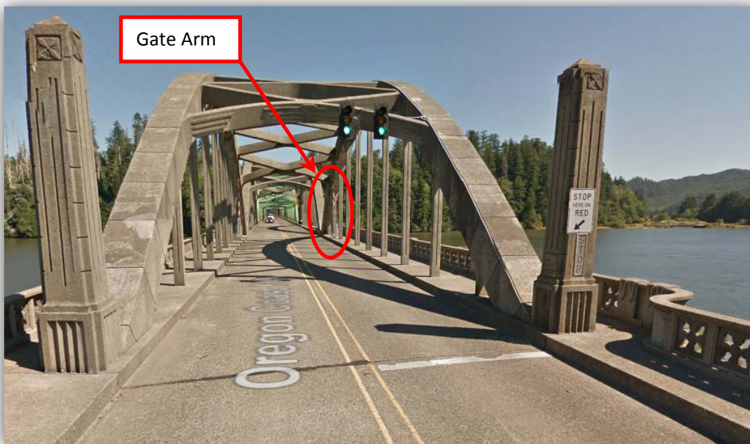
Figure 23-8 | Example of Existing Warning Gate Arm Located Downstream from Signal Indications
