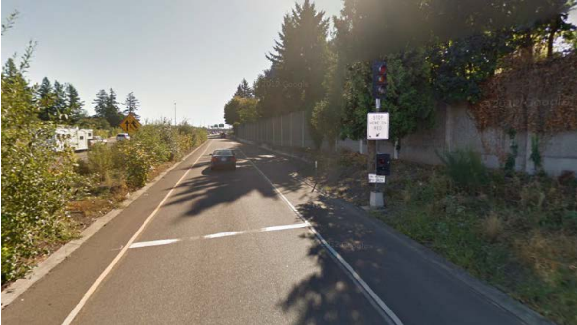
Figure 13-5 | Ramp Meter Pedestal Mounted Assembly Example – Controlling a Single Lane of Traffic
