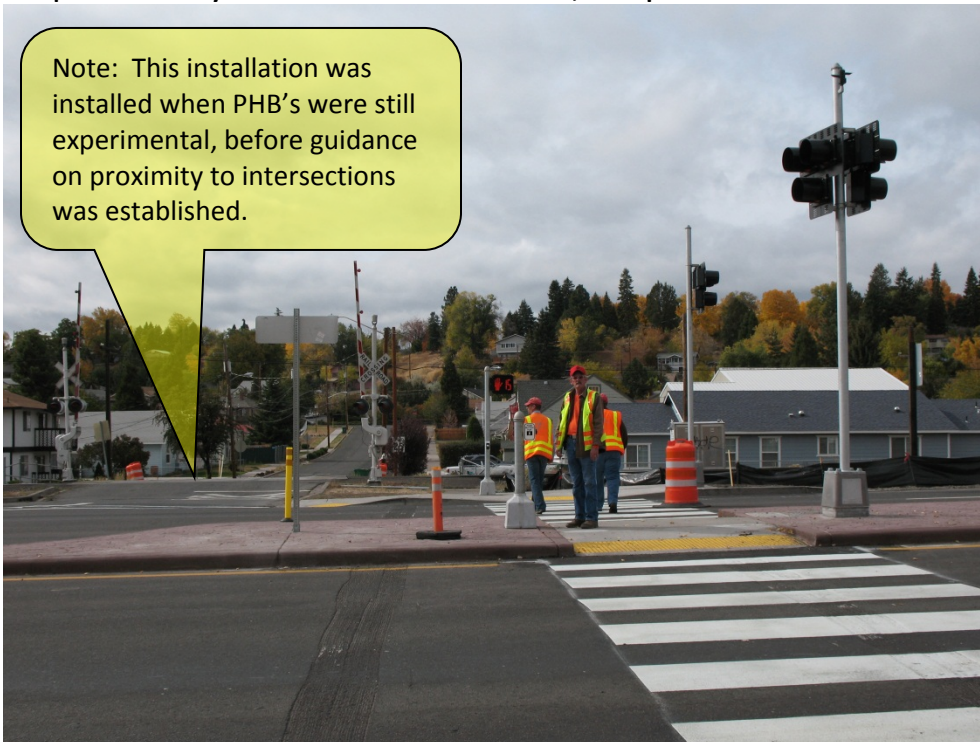
Figure 12-21 | Pedestrian Hybrid Beacon – Ground Mounted, Example 2
