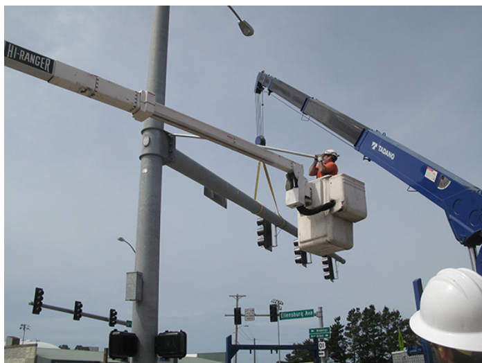
Bolt Tightening with Cheater Bar (May be difficult to achieve proper tensioning)
