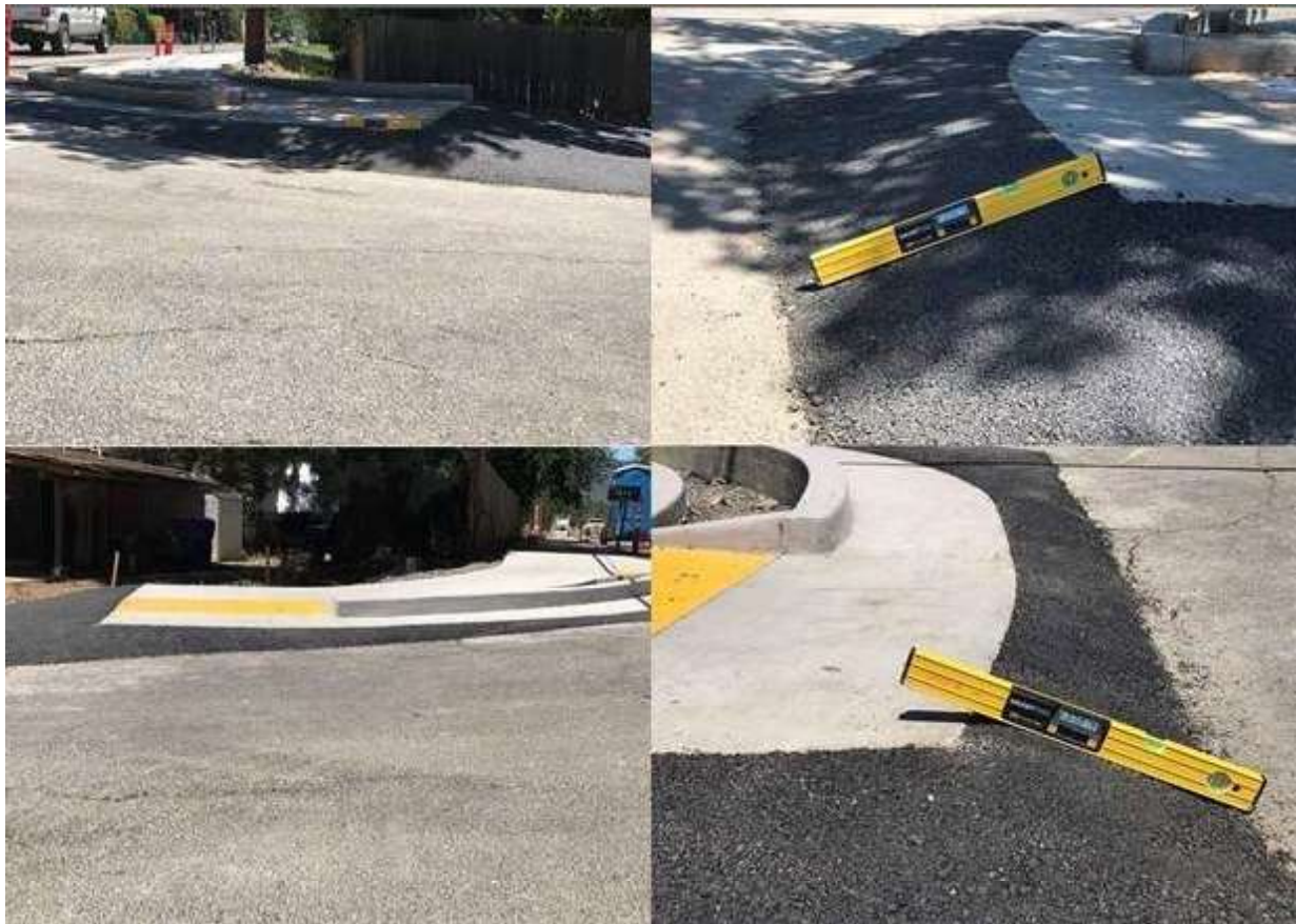
Examples of a non-accessible connections to the road.
