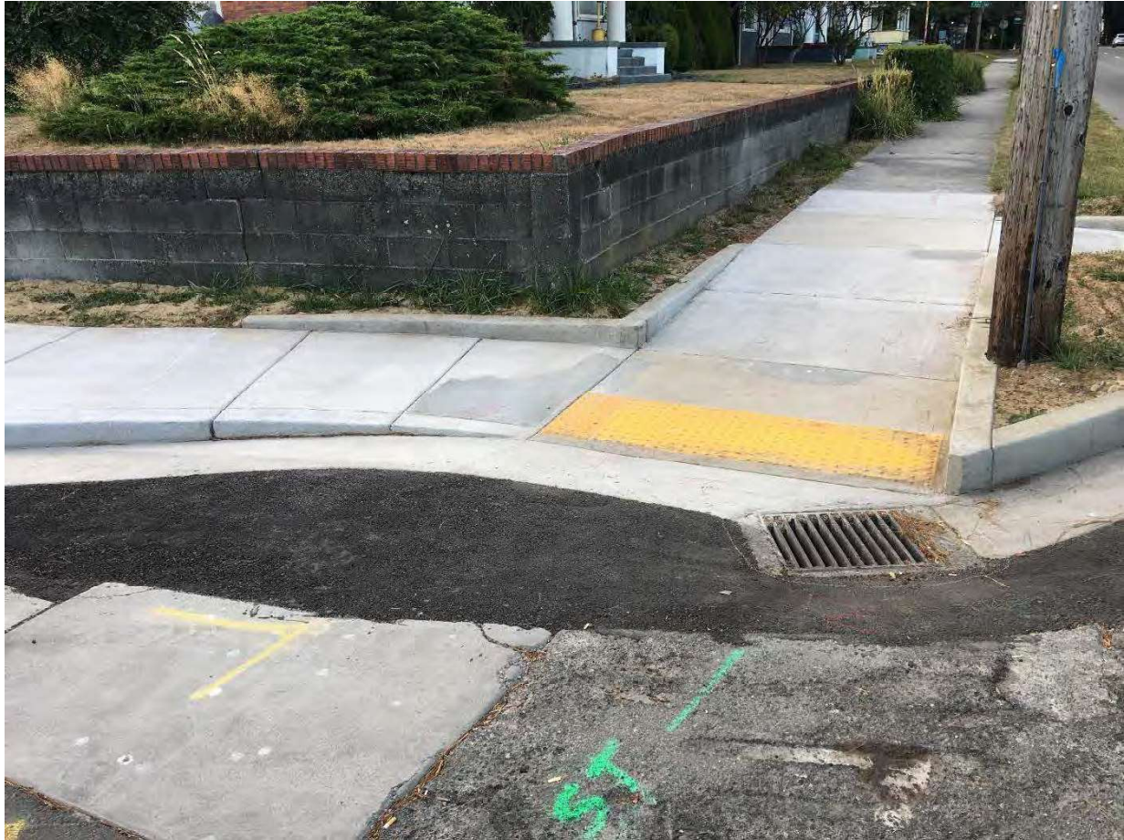
Inlets Photo 1: Inlet within the pedestrian access route at the ramp opening causing failure.
