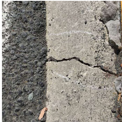
F/W issues Photo 4: Cracking that is not the result of concrete curing and creates barriers to access will result in failure.
