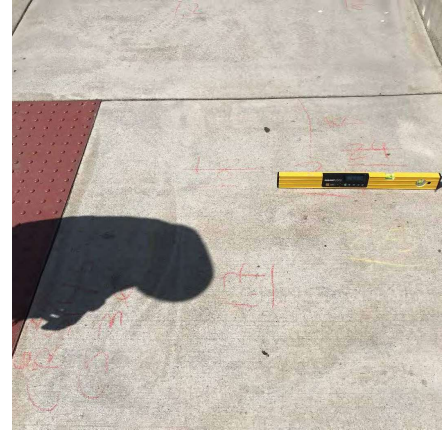
F/W issues Photo 2-2: A close up of "F/W issues Photo 2-1" showing an isolated area on the turn space where slopes are over the maximum of 2.0%.
