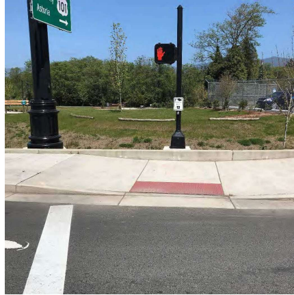
F/W issues Photo 2-1: A newly constructed parallel ramp with isolated slope issues on the turn space.
