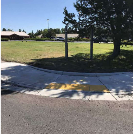
F/W issues Photo 1: A newly constructed parallel ramp with a ramp run 3 that is crumbling at the curb.
