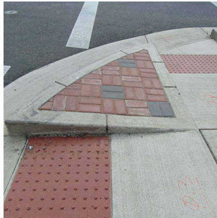
Drop Off photo 2: Curb Ramp designs that use return curb creating a triangle piece between the two ramp positions requires a non-walkable surface to be installed.
