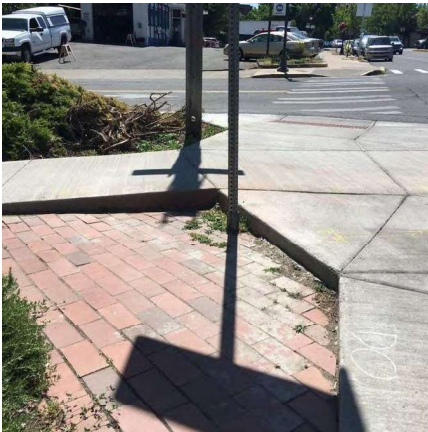
Drop Off Photo 1: Vertical discontinuities within curb ramp proximity limits will result in failure.
