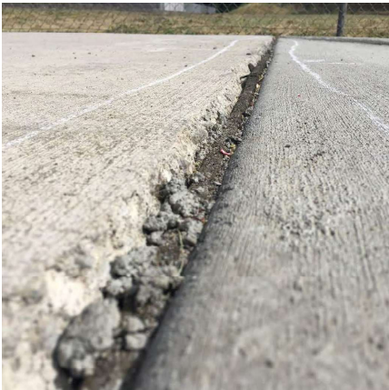
F/W issues Photo 3: A photo of a joint creating a lip issue between new and existing concrete. Lips
