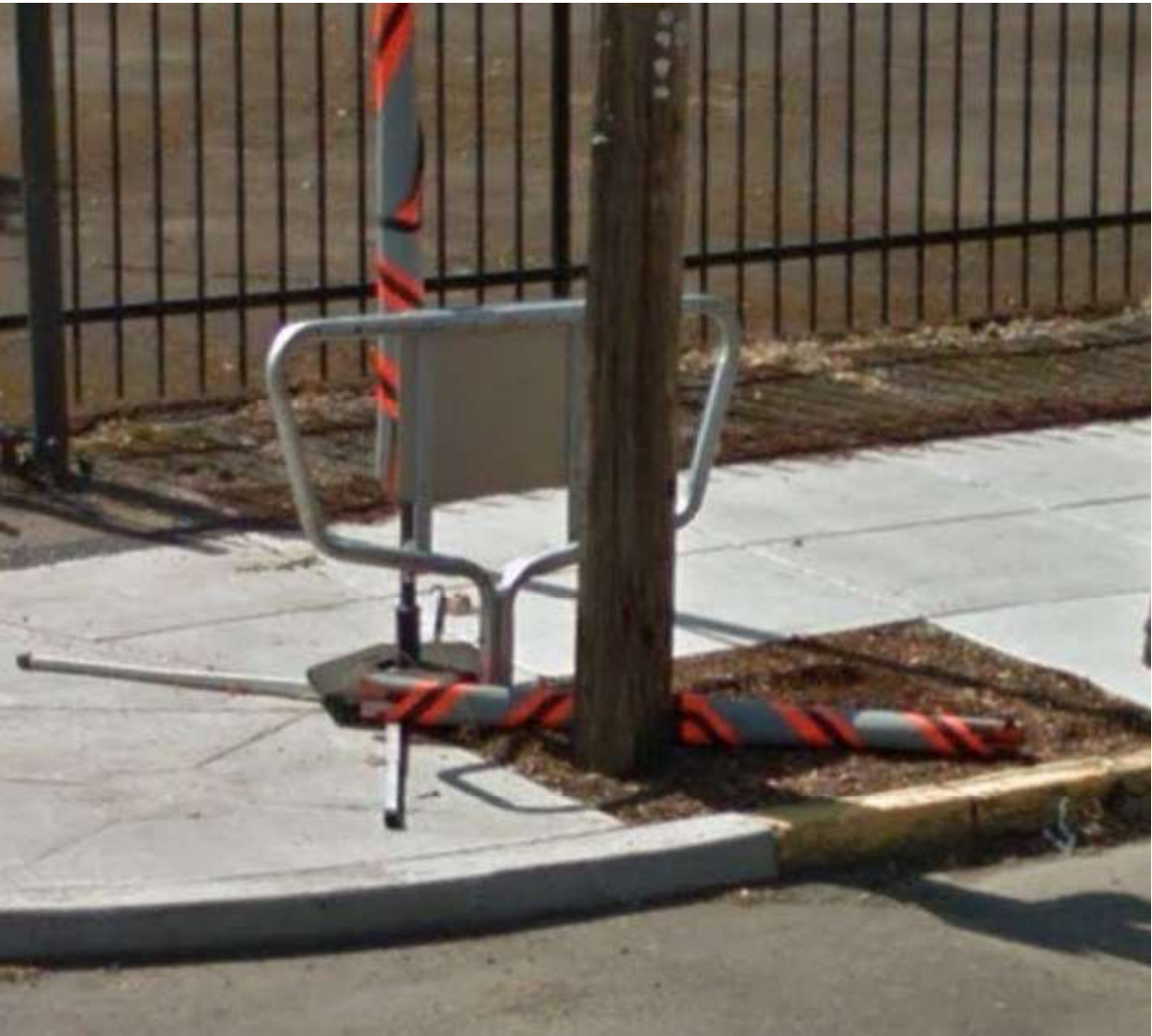
Example 2: of Incorrectly installed crosswalk closure support
