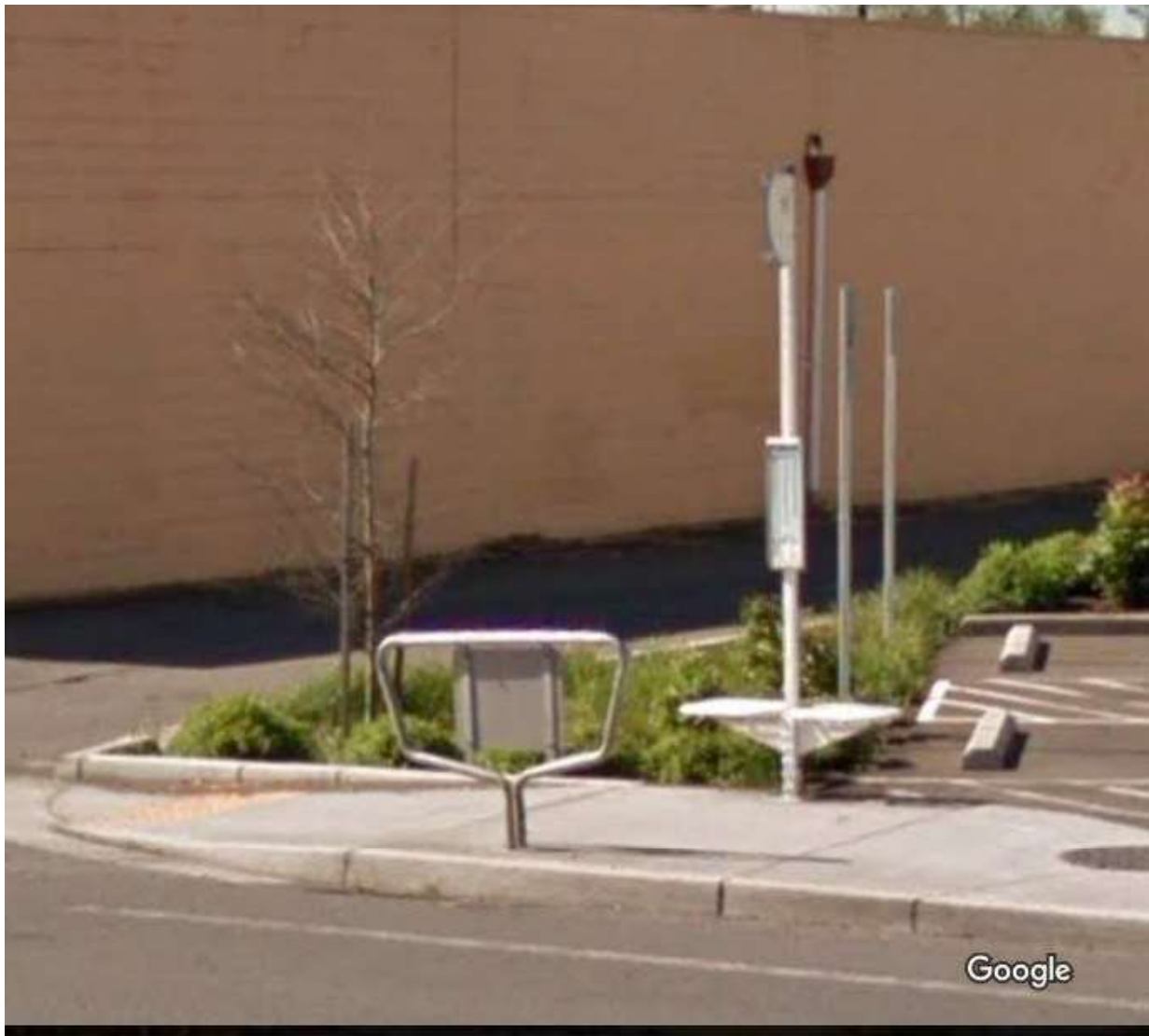
Example 3: Missing Sign on a crosswalk closure support
