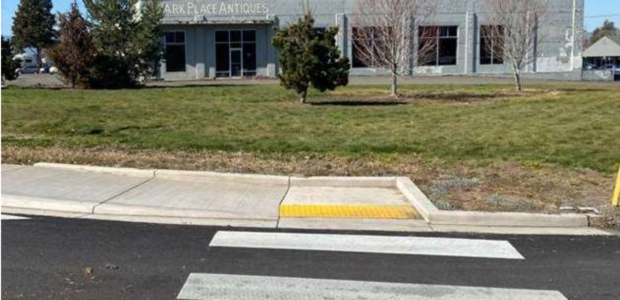
This looks like a parallel curb ramp with a ramp run missing. Use the Unique Curb Ramp Inspection form.
