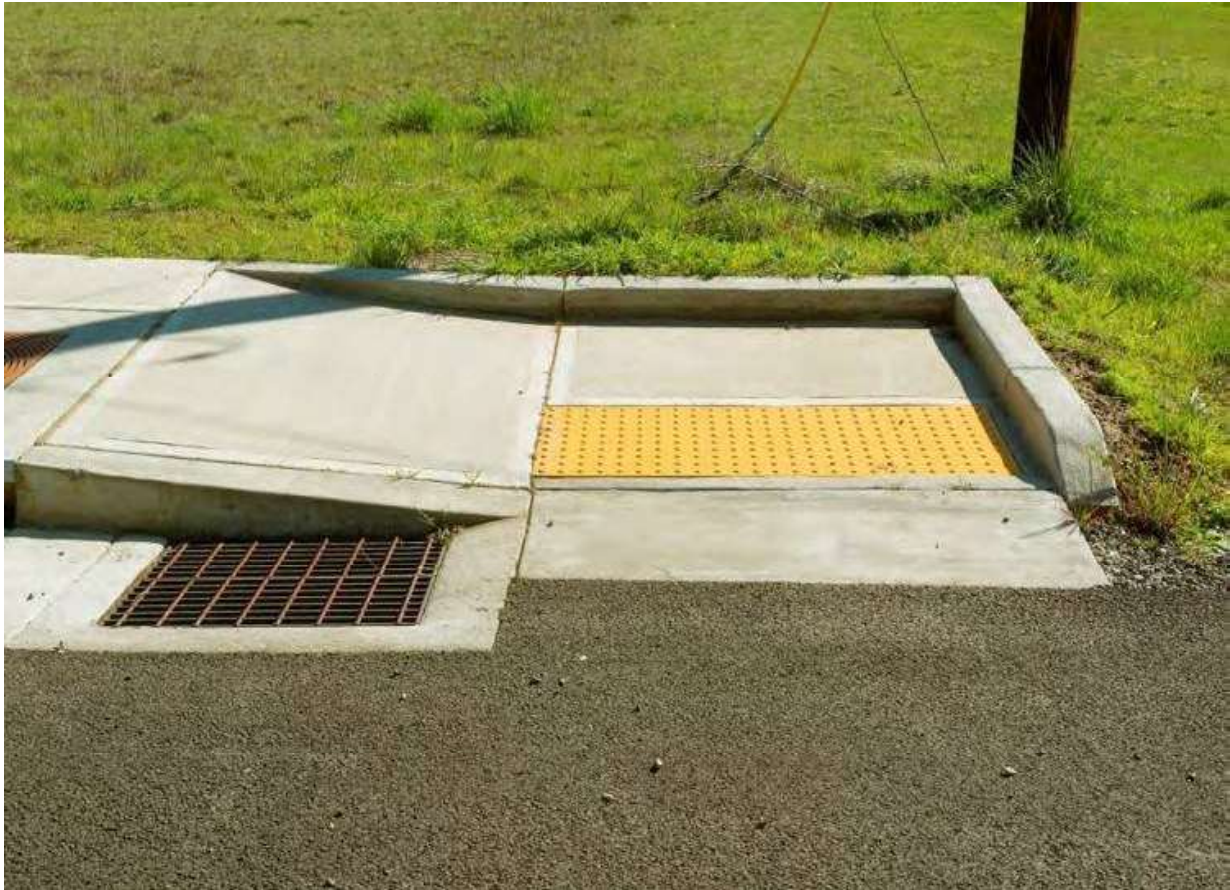
A One-Sided Parallel Ramp is Considered a Unique Design Style Curb Ramp
