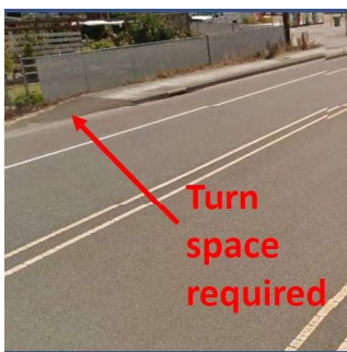
End of Walk Curb Ramp that Requires
