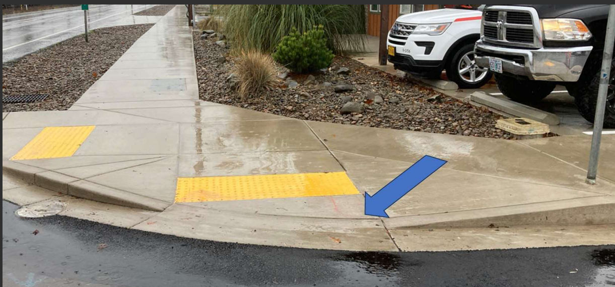
Improperly Installed Detectable Warning Surface. Pedestrian with Visual Impairments Could Miss Detectable Warning
