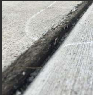
Expansion Joint Lip Failures
