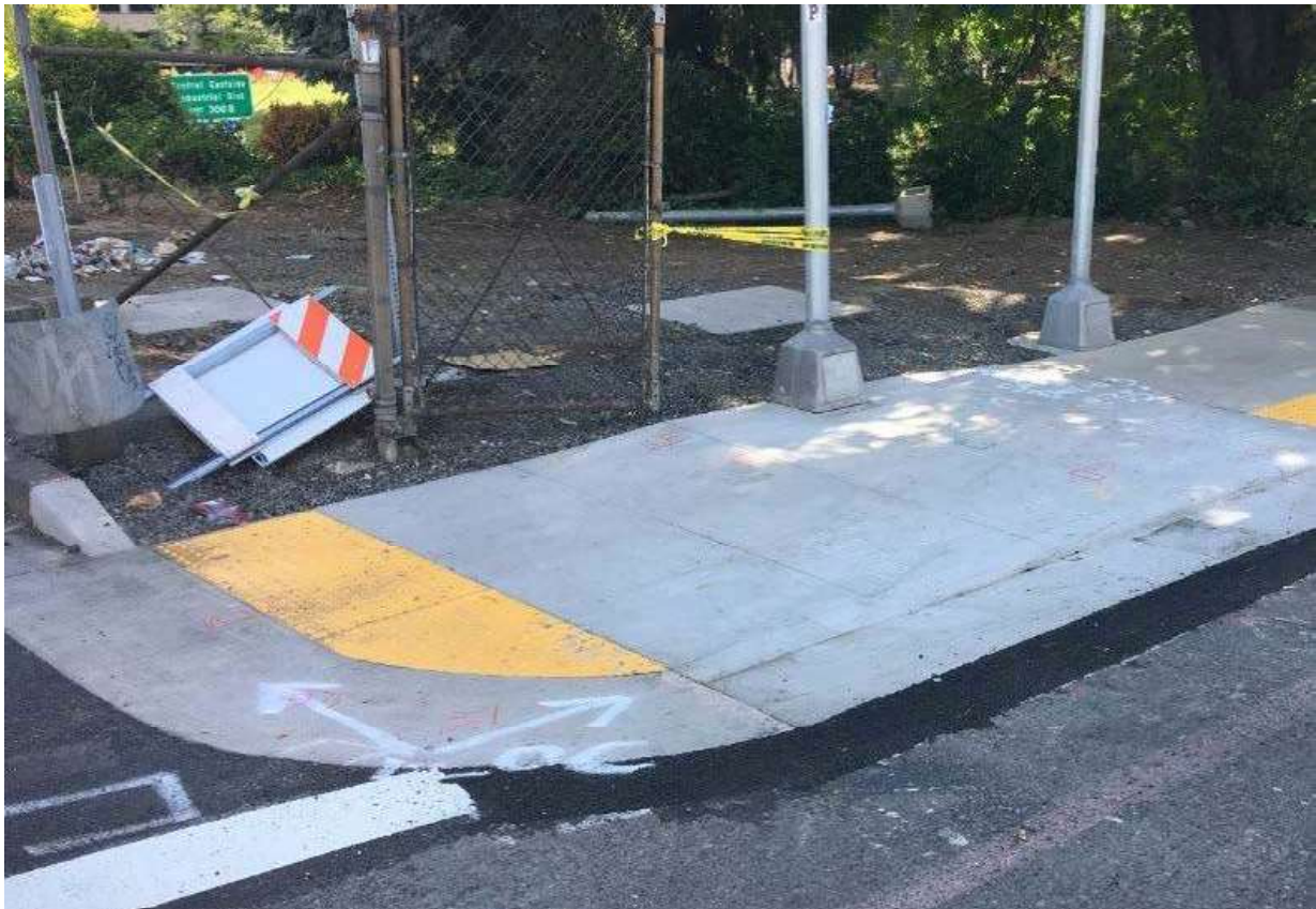
Improper Detectable Warning Surface Cut To fit The Curve of The Curb
