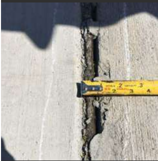
Expansion Joint Gap Failures
