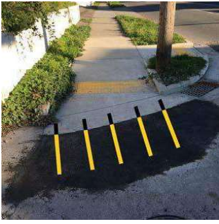
Correct Placement of Smart Level for Measuring Running Slope of New Asphalt Connection
