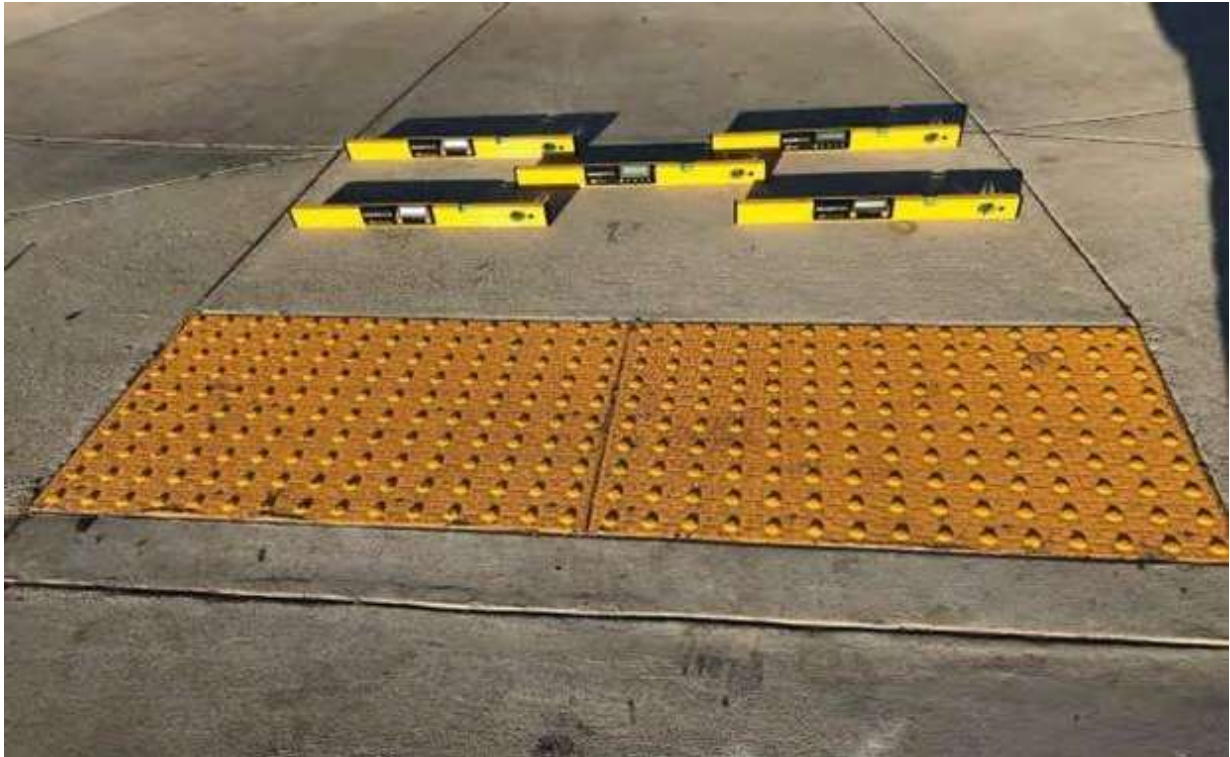
The Photo Illustrates an Example of Cross Slope Level Placement on a Ramp Run
