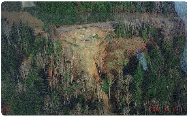
Figure B8: Complete roadway failure on U.S. 30 east of Clatskanie, 1996. Note the section of undermined pavement
