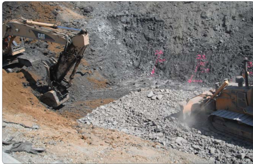
Figure B16: Constructing a shear key and buttress is one of the most common methods for stabilizing larger landslides due to the generally high resisting forces introduced, their ability to drain water, and their capacity to arrest slide movement. This is a more costly approach to slide mitigation, but it is one of the most effective. The shear key is simply a notch cut through the slide surface and into stronger, more resistant soil or even rock. This notch is fitted with a perforated pipe drain system and then backfilled with compacted stone embankment to form the "key" that provides shear resistance to sliding. The buttress constructed on top of the shear key provides strong material at the toe of the slide and additional mass to resist sliding; it also forces the key downward and increases its shear resistance. The dimensions of the shear key and buttress are dictated by the size of the landslide. In some cases, shear keys and buttresses are used independently, depending on need and site conditions. When buttresses are used without a shear key, they are known as counterbalances.
