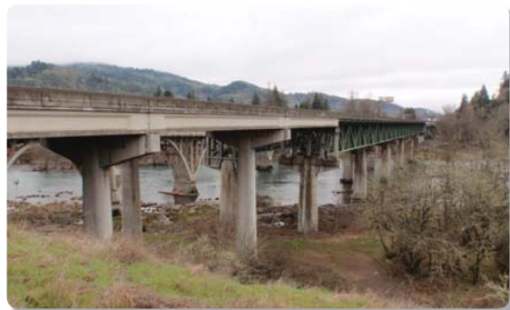
Figure B4: North Umpqua River (Winchester) Bridge, one of the state's many large bridge structures. The repair or replacement of such bridges after a subduction zone earthquake will be both challenging and time-consuming.
