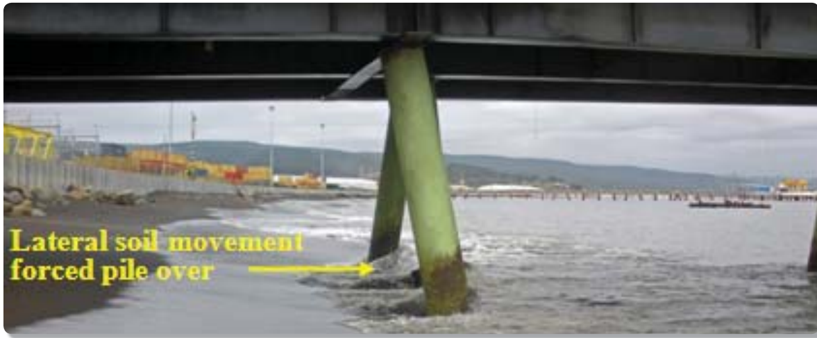
Figure B13: Strengthening the foundation or soil mitigation will prevent damage to the bridge substructure caused by liquefaction and lateral spreading.
