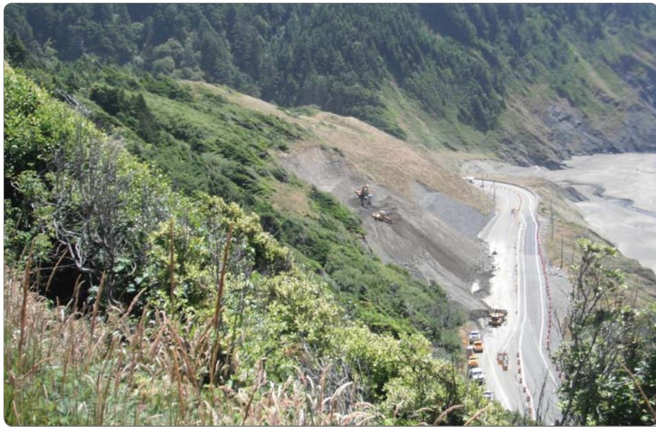
Figure B18: Steep slopes, coupled with weak materials and water, are one of the principle causes of landslides. Decreasing the angle of a cut slope is a common method used to decrease the driving forces acting on the slope or landslide. Not only can the head of a slide or unstable slope be unloaded, but a more stable geometry can be created by the flatter slope configuration. The angles at which cut slopes can be constructed are a function both of the material's strength and height and of any groundwater seepage in the slope. Rock slopes can be cut almost vertically, while weak clay materials must sometimes be cut as shallow as four feet horizontally for every one foot of height. Flatter slopes are more resistant to ground shaking in an earthquake, but are limited by the amount of adjacent property that must be acquired to construct them.
