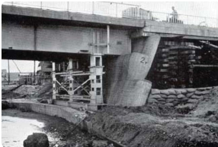
Figure D1: Bridge pier damage resulting from liquefaction and lateral displacement of foundation soils (Yachiyo Bridge, 1964 Niigata, Japan)
