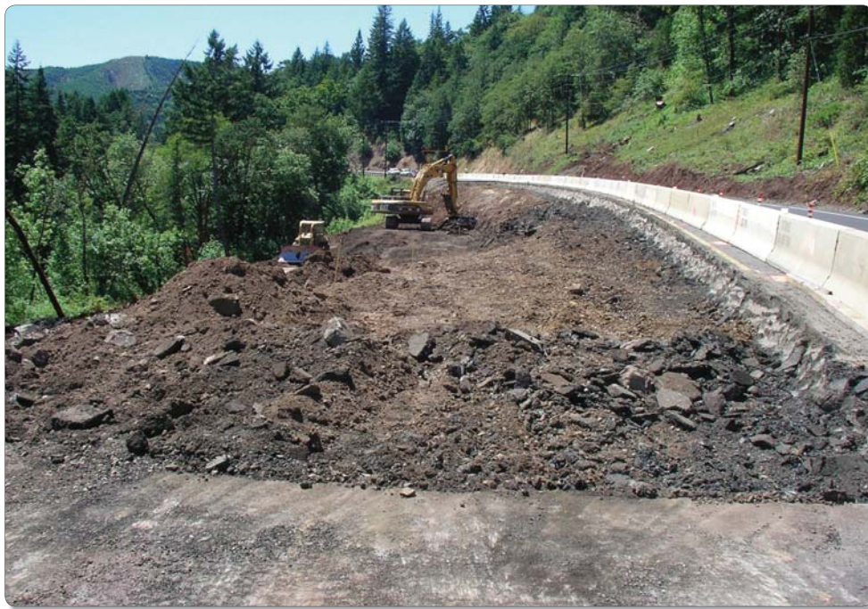
Figure B17: One of the simplest methods for stabilizing a landslide is to remove, or “unload,” as much of the mass of materials pushing down on it as possible. The more weight that can be removed from the top (head) of the slide, the more stable it becomes, and also the more resistant to seismic forces and effects. Slide unloading is used where the vertical alignment of the roadway can accommodate a lowered grade and in cases where the slide occurs above the road. This method is generally a low-cost approach to slide stabilization, and some further slide movement is expected after construction, although at a much lower rate and magnitude.
