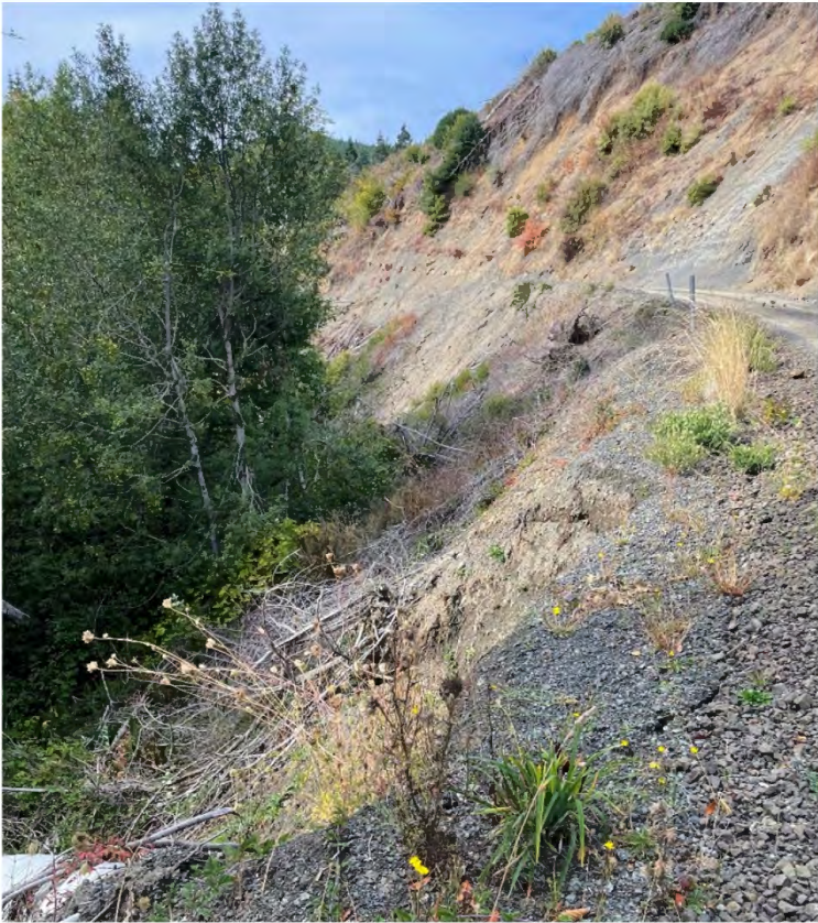
Figure 3. Example of a road segment with perched fill that presents a significant hazard to a fish-bearing stream.
