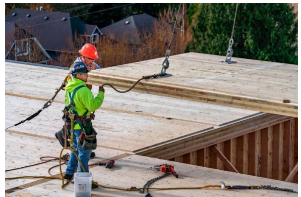
A construction crew installs a cross-laminated timber panel (Source: Marcus Kauffman, Oregon Dept. of Forestry)
