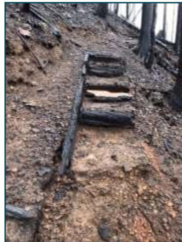
Image of trail damage
