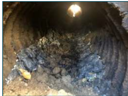
Image of a burned out culvert
