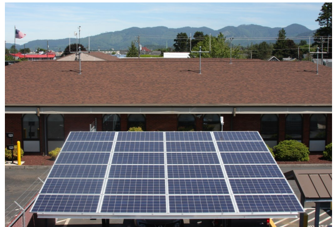
Tillamook PUD's headquarters has solar on site.
