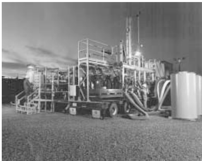
Carbon tetrachloride vapor extraction system
