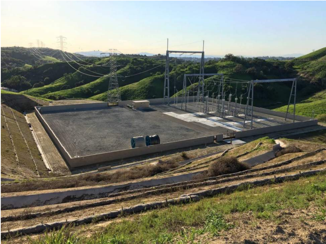
Figure 9: Example 500 kV Transition Station
