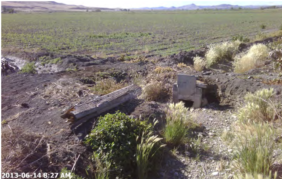
Photo P334. Feature MA_TM_483. Irrigation ditch with a cement control structure in the center of the image. Looking East, in Malheur County. 6/14/2013 8:24. Latitude 44.076207. Longitude -117.28519.
