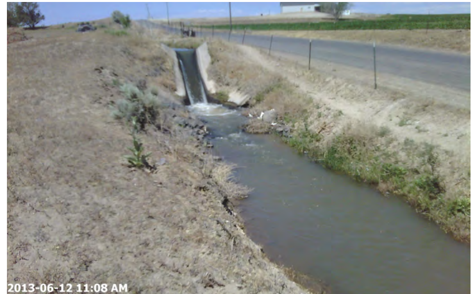
Photo P335. Feature MA_TM_465. Cement spillway in the center of the image with the paved road to the right. Looking West, in Malheur County. 6/12/2013 11:04. Latitude 44.068933. Longitude -117.309946.
