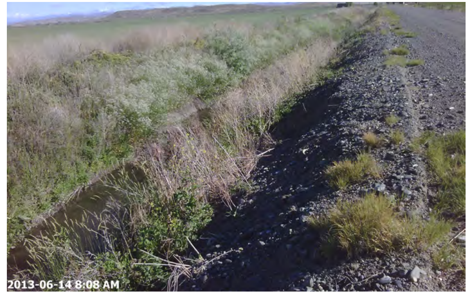
Photo P333. Feature MA_TM_482. Irrigation canal running adjacent to a gravel access road. Looking North, in Malheur County. 6/14/2013 8:07. Latitude 44.076409. Longitude -117.285293.
