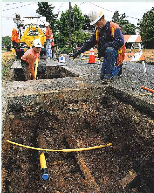
Utility Assistant Bryan Baxter (background) feeds new polyethylene pipe to Pipe Joiner Chris Wiles (in ditch), who inserts it into 100-year-old cast iron pipe as part of the Company's replacement of its low-pressure distribution system. Distribution Crew Leader Hayden Golden directs the process.
