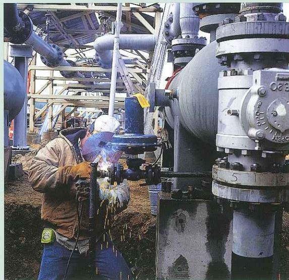
Bert Kilcrease, a contract employee from Rockford Corp., completes the tie-in of the newly developed Reichhold Pool to NW Natural’s underground natural gas storage system at Mist.
