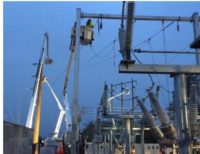
Grid Edge Demonstration Project in Eugene Photos courtesy of Eugene Water and Electric Board
