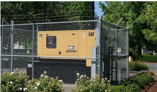
The Oregon Department of Energy office in Salem has a 300-gallon diesel backup generator that can provide power to critical agency equipment for about 24 hours in the event of an outage or emergency.
