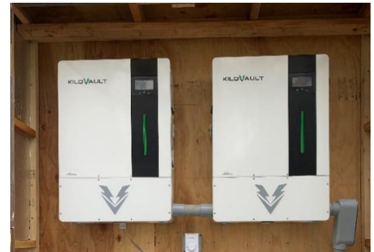
This residential battery storage system stores energy generated by rooftop solar panels.
