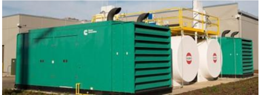
Diesel generators and fuel storage tanks. Photo: Portland General Electric
