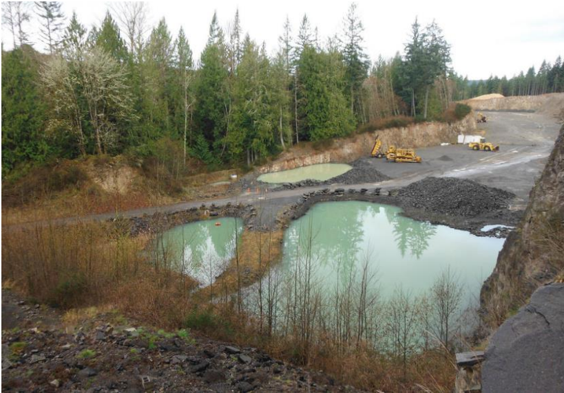
Stormwater control system at Graves Quarry in Molalla
