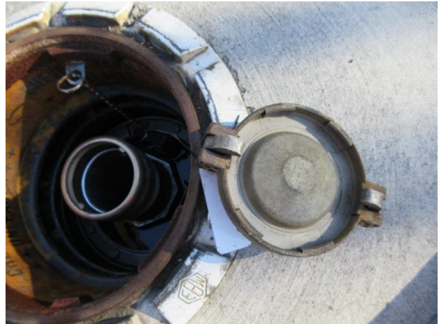
(AQGP-22 & 23) Dust Cap is broken
