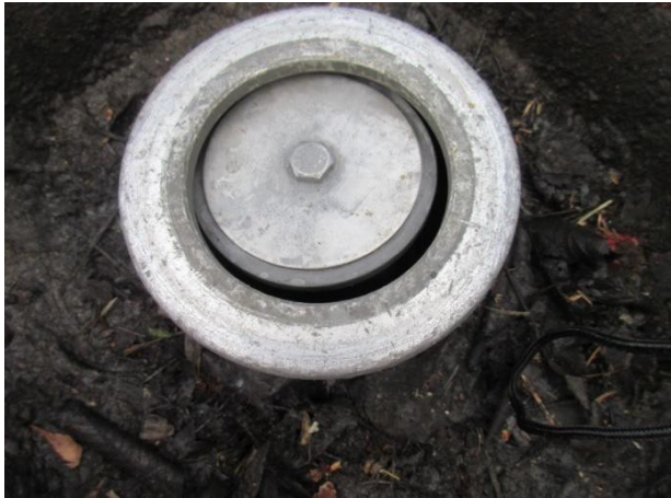
(AQGP-22 & 23) Poppet valve not sealed
