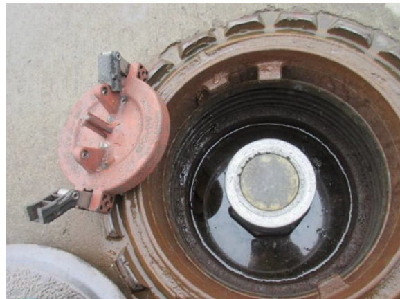
(AQGP-22 & 23) Dust Cap/Fill Tube: No gasket seal
