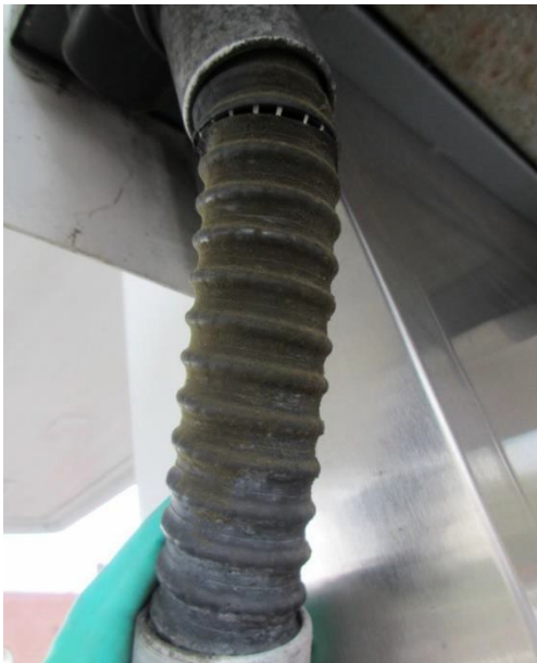
(AQGP-23) Balance whip hose is torn
