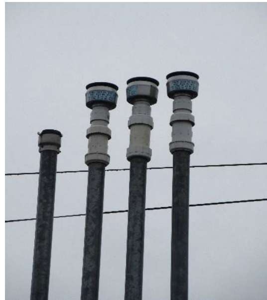
(AQGP-22 & 23) This picture shows three PV valves, one for each gasoline tank on site, and one open atmospheric vent (left) piped to the diesel tank. Note that one PV valve is acceptable for multiple gasoline tanks if the piping is manifolded together. All Stage 2 permitted sites require PV valves for gasoline storage tanks.
