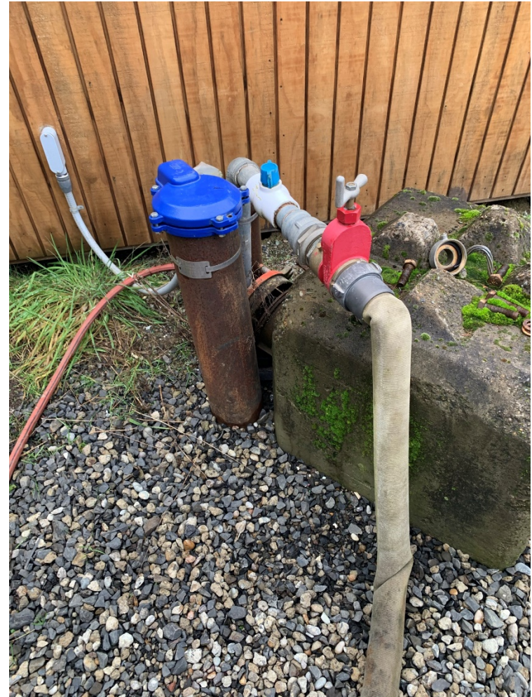
A close-up view taken the week before sampling shows the wellhead with a gate valve and a 2-inch flex hose attached to the well. The flex hose was used to purge the well prior to sampling.
