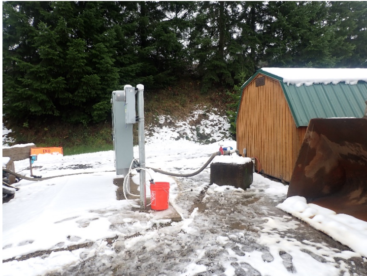
The on-site water well is located in the northeastern part of the Westside Rock quarry. The well head is shown next to the shed. The control panel and pressure tank were located inside the shed.
