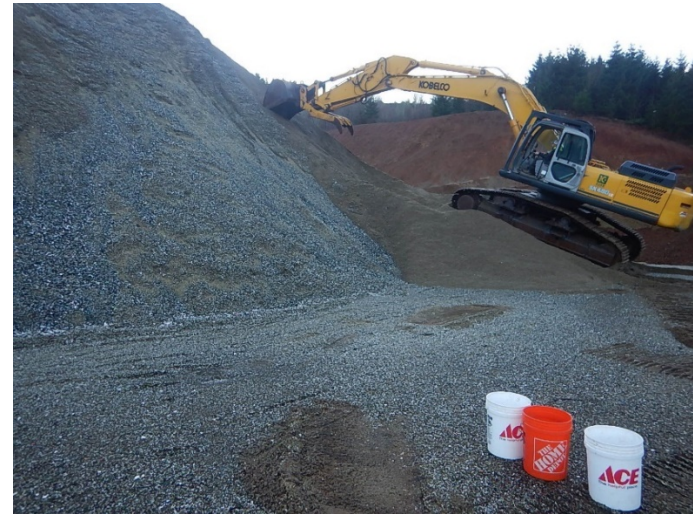
West Side Entity provided equipment and an operator to assist with sampling efforts within DU01. 60 subsamples (increments) of material were collected from the sides, top, center, and base of the stockpile with the assistance of the track hoe.
