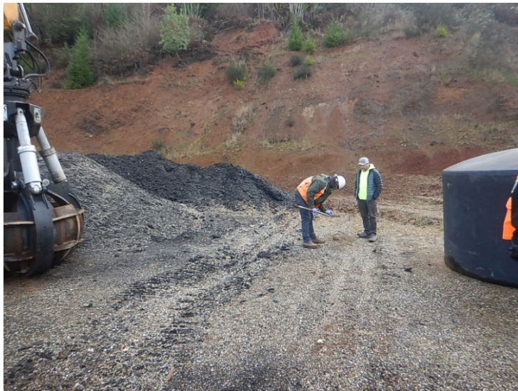
View of the Type 2 material placed as haul road cover and also forming berms surrounding parking/storage areas (DU02).
