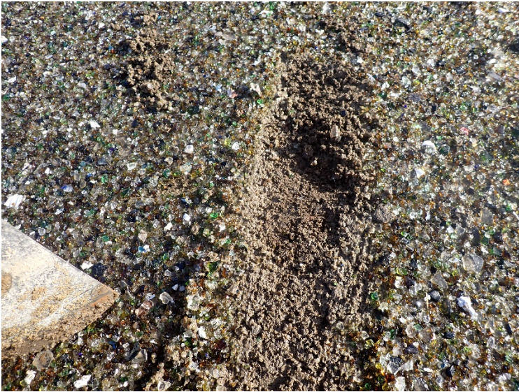
Close-up view of glass cullet placed as cover on haul roads within DU02.
