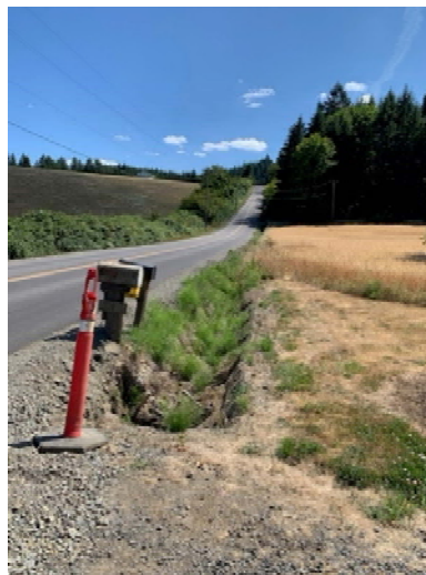
View south along Hergert Rd ditch from the Husin Driveway entrance. (August 7, 2020)
