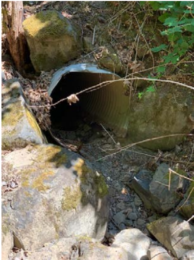
View of culvert inlet C1, hydraulically down-gradient of impoundment structure, showing absence of sediment and iron staining. (August 7, 2020)
