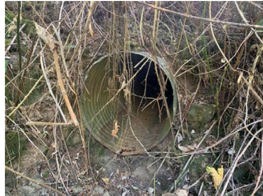
View of outfall of lower culvert showing absence of sediment and iron staining. (August 7, 2020)
