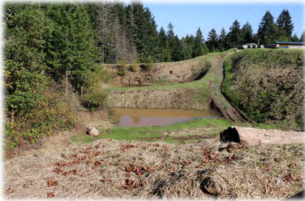
Pond #1 with vegetated side slope and armored with rip rap at inlet and outlet
