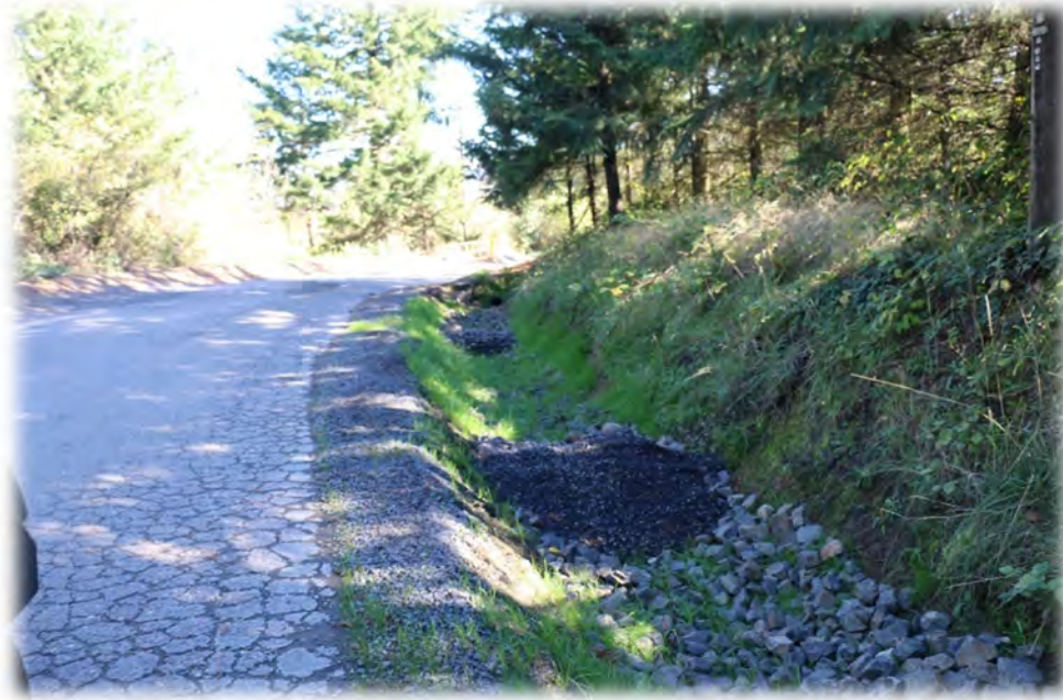
Vegetated swale with armored check dams and bottom along paved entrance
