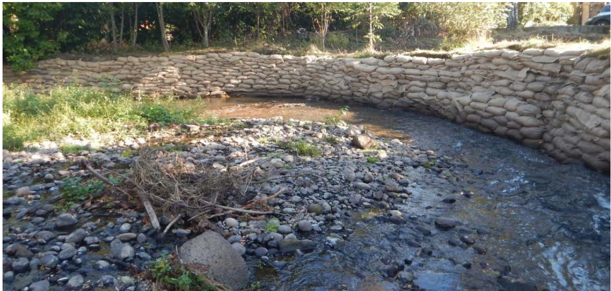
Figure 3b: Scarp at Johnson Creek Oxbow after temporary jute bag installation (Inter-fluve, 2017)
