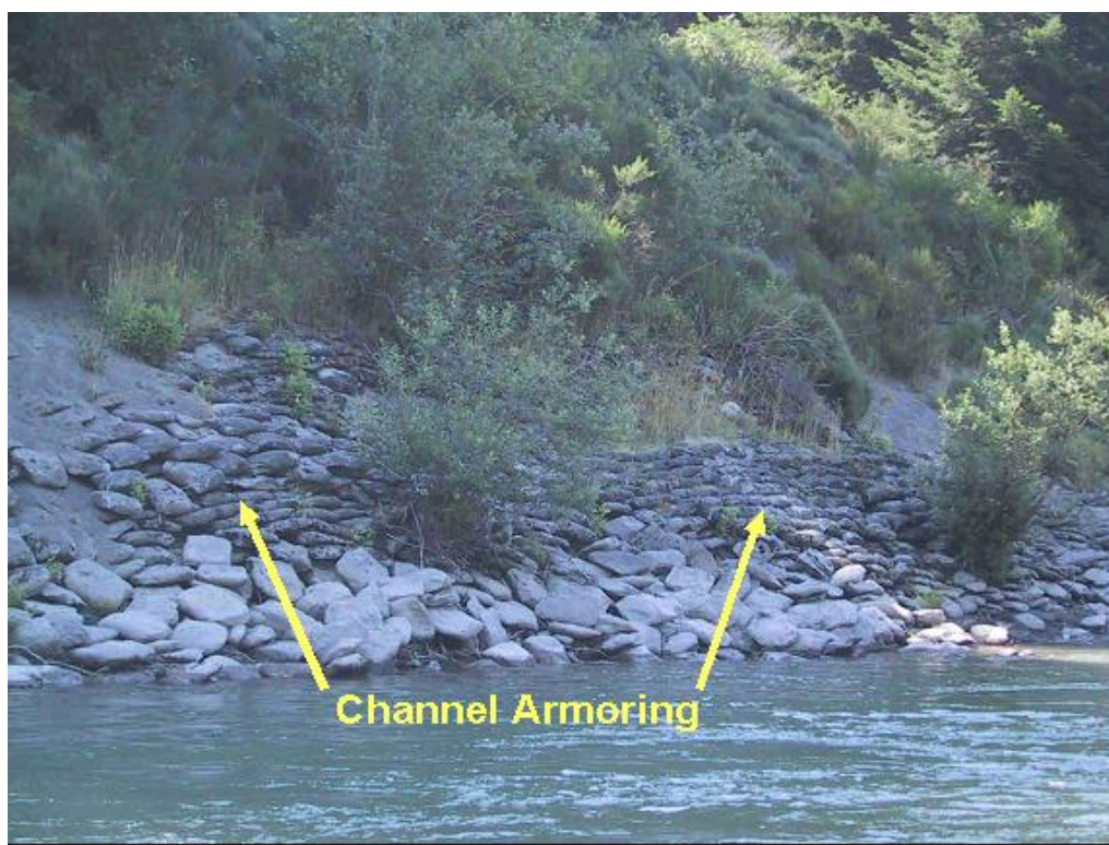
Concrete Channel Armoring along the Sandy River near Oxbow Park
