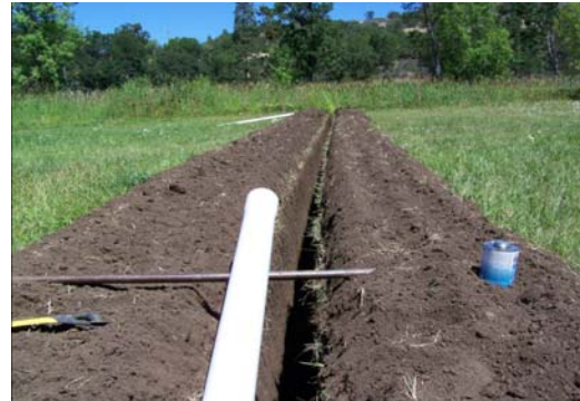
Push up dams along Little Butte Creek are removed as pumps and irrigation lines are installed
