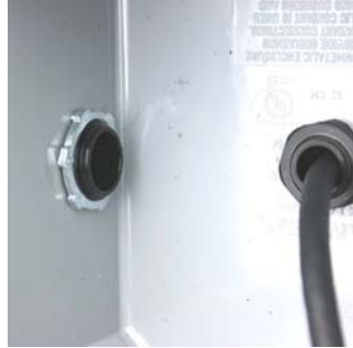
Nut on back side of conduit connector
