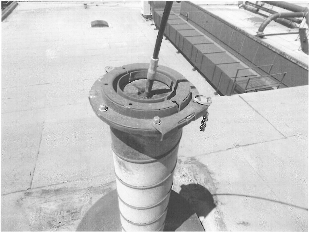
Cleaning cap installed
