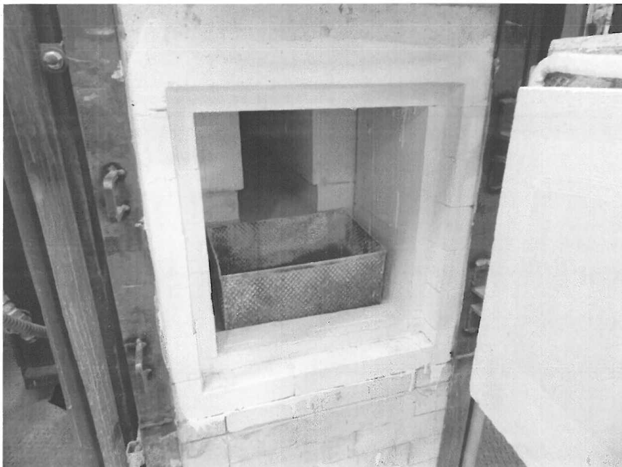
Stack cleaning particulate catch box
