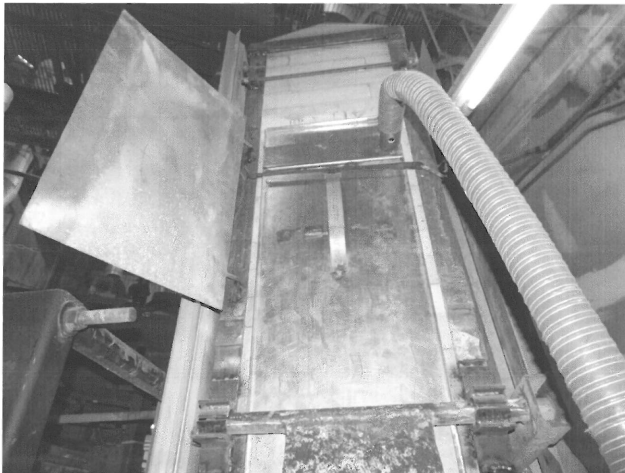
Damper opening cover with vacuum hose attached
