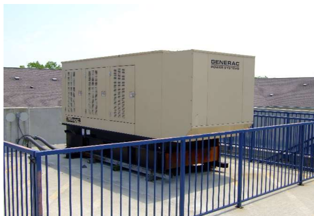
2020 - Emergency Standby Generator Total Project Cost: $166,667 ODAV COAR Grant: $150,000
