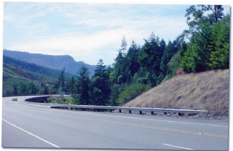
Taking an inventory of traffic barriers was the first step in addressing a standards upgrade.
